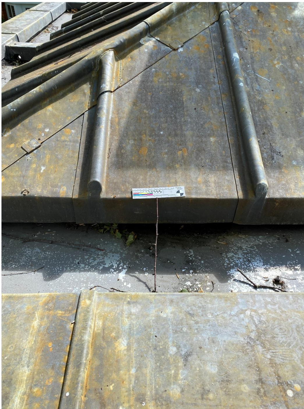
SAL 8 Discolouration of the lead material to the dwelling. In the top left of the image, the normal state of the lead material.
