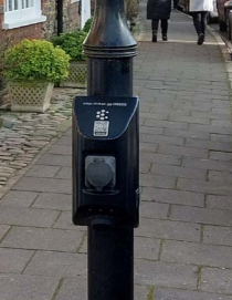
FIGURE 215 STANDARD LIGHTING COLUMN WITH EV CHARGING POINT
