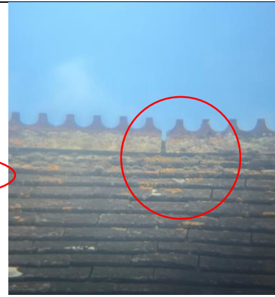
Figure 4: Missing mortar between the ridge tiles.
