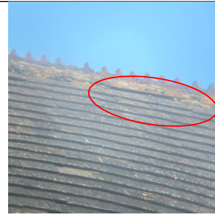
Figure 5: Gaps between the ridge tile and roof tiles.
