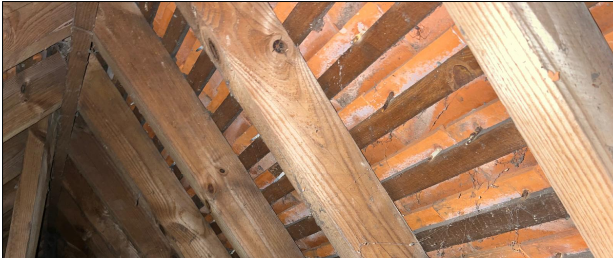
Photo 2: Lack of roof lining and insulation in the eastern section of the loft.
