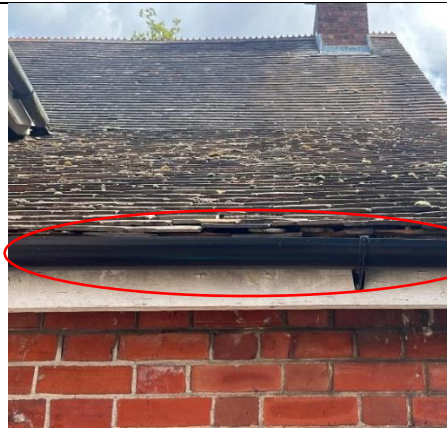
Figure 3: Lifted roof tiles on the western sloped roof.
