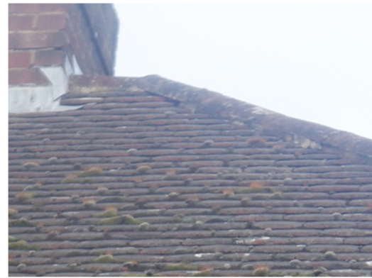
Photograph 4. Section of mortar missing from a hip tile to the front of the house.
