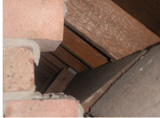
Photograph 12. Gaps in the brickwork at the gable.
