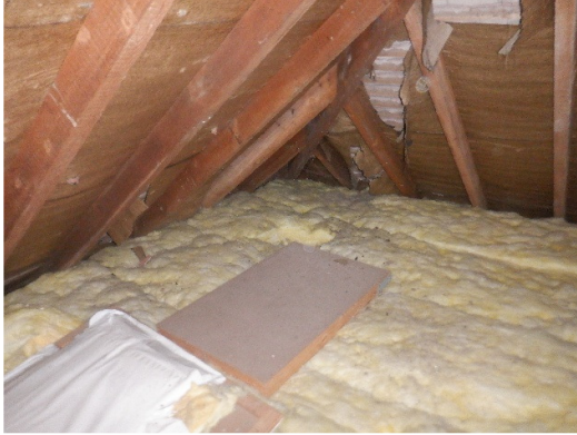
Photograph 11. Eaves open in places.
