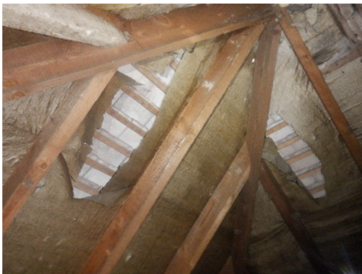
Photograph 8. Large tears in paper backed felt.
