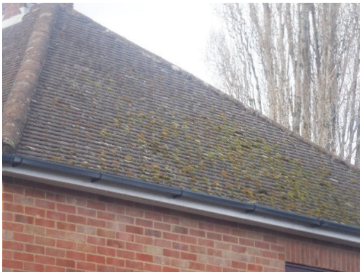
Photograph 3. Flat moss covered roof tiles at the southern side of the house.
