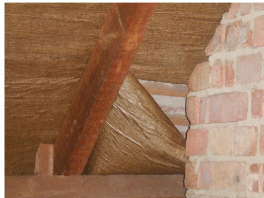
Photograph 9. Large tears in paper backed felt..
