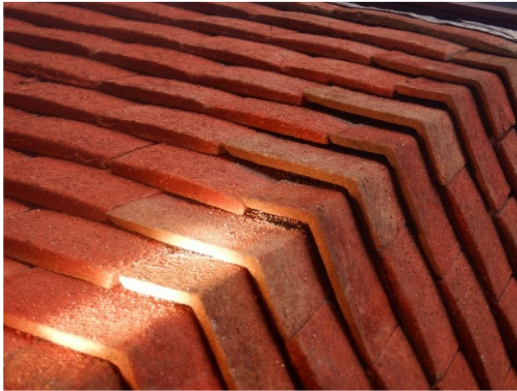
Photograph 7. Gaps behind the ganging tiles on the bay window.
