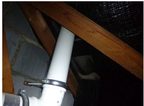
Photograph 13. Boiler at western gable end (roof void).
