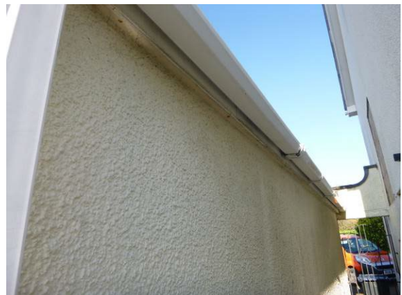
Photograph 9. Tight fascias on garage (eastern elevation).
