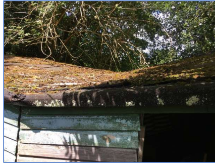
Photo 58 Dilapidated structure (B5)
