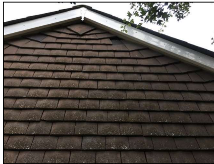
Photo 66 Bird nesting behind slipped tile
