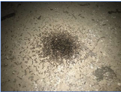
Photo 53 Cluster of bat droppings pile 1 (B3)
