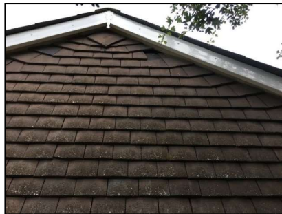
Photo 42 Missing wall tile (B2)
