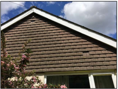
Photo 37 Slipped tiles (B1)
