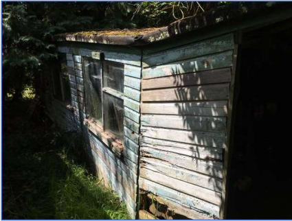
Photo 57 Dilapidated structure (B5)
