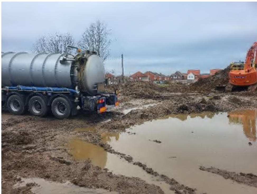
Plate 2 – Vacuum tanker onsite to remove surface water
