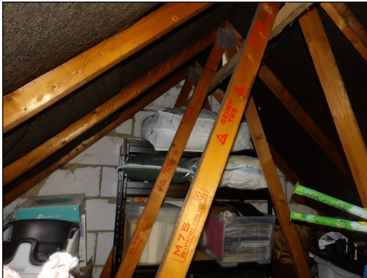
Figure 11. Example of loft space and bitumen felt in property. 190 Hurricane Way, Woodley. 19.08.25
