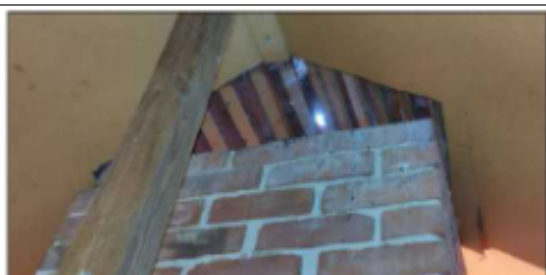
Figure 9 – Roof void above extension to the rear, with no insulation found on top of bitumen felt
