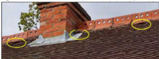
Figure 13- showing missing tiles and gaps along the ridge
