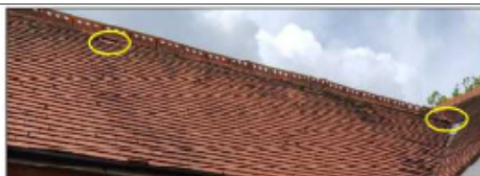
Figure 14- showing missing tiles and gaps along ridge on rear extension
