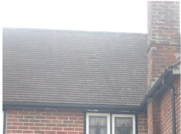
Photograph 4. Mostly tight roof tiles; broken roof tile, offering no roosting opportunities (rear elevation).
