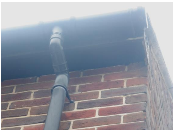
Photograph 8. Timber soffit tight to brickwork (rear elevation).
