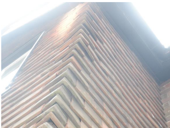
Photograph 10. Lifted and uneven hanging tiles on front gable (front elevation).
