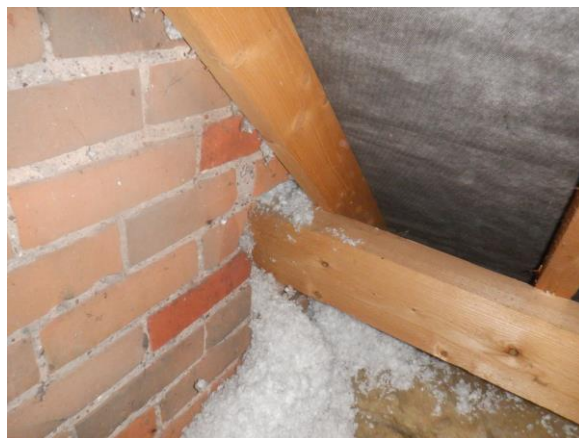
Photograph 16. Shredded cavity insulation coming out of the rear gable around the timber beams (roof void).
