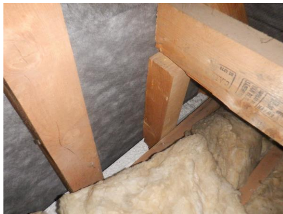
Photograph 13. Eaves blocked with polystyrene boards (roof void).
