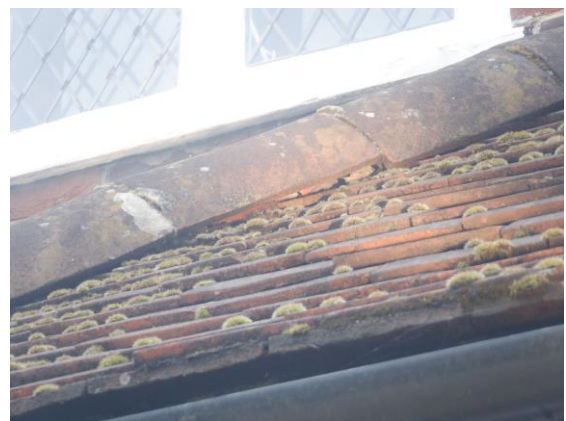
Photograph 7. Missing mortar under the hip of the single-storey roof (rear elevation).
