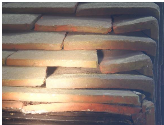
Photograph 11. Small-sized bat droppings observed under lifted hanging tile (front elevation).
