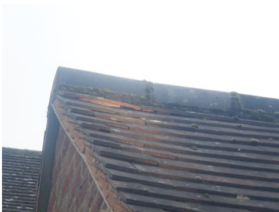
Photograph 6. Lifted verge tiles; no suitable gap observed (rear elevation).
