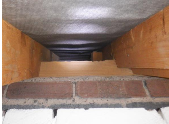
Photograph 18. Gap above brickwork wall (garage loft).
