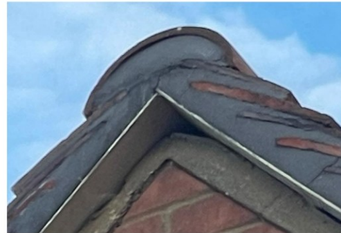
Missing mortar at AP1
