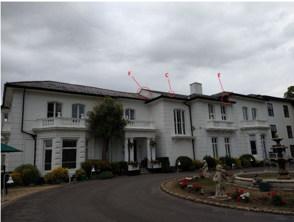
Photograph 2: South eastern elevation of B2 showing location of features C (lifted tiles), E (missing mortar) and F (rotten weather board and lifted lead flashing).
