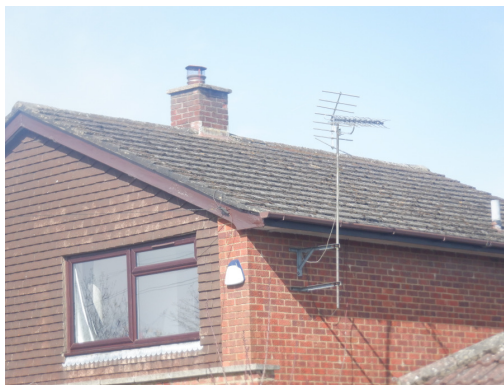
Photograph 4. Tight/flat plain roof tiles and gaps in ridge tile mortar
