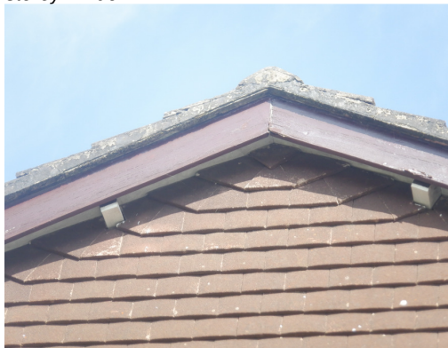
Photograph 8. Gaps between soffit boxes and hanging tiles (south elevation)
