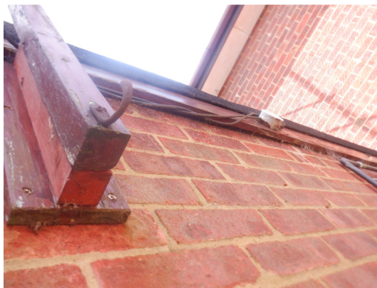
Photograph 13. Superficial gap in bargeboards northern side of garage building
