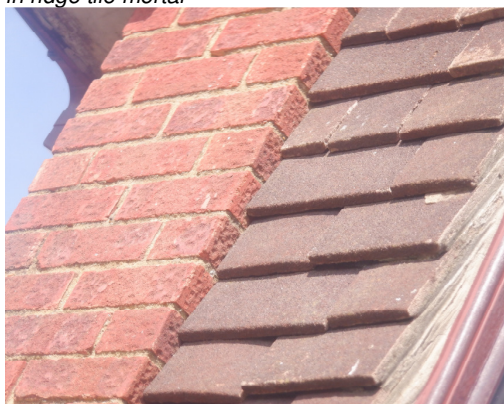
Photograph 6. Gaps in east side of front second-
