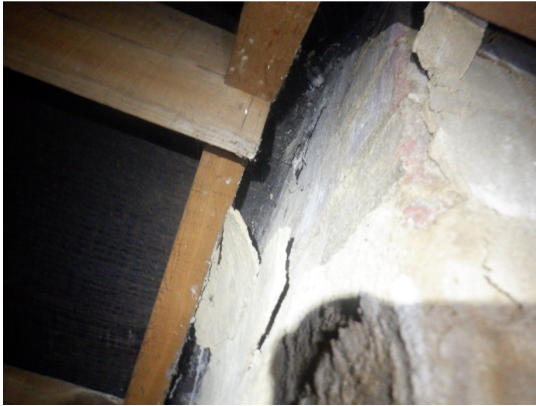
Photograph 20. Crumbling render around chimney brick in centre of the loft void and tight to bitumen roof felting.
