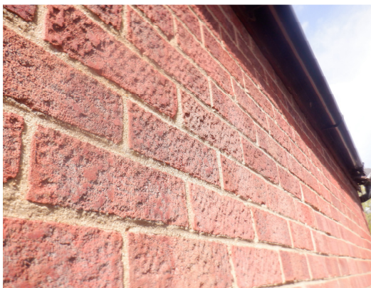
Photograph 12. Tight bargeboards around garage building eastern side of property.
