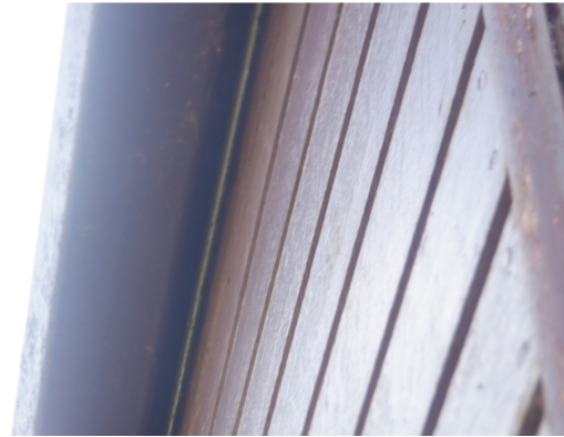
Photograph 16. Flat timber cladding tight to rubber flat roof on existing rear extension.
