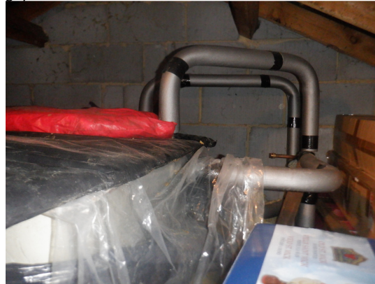
Photograph 21. Covered water tank to the north of the loft void.
