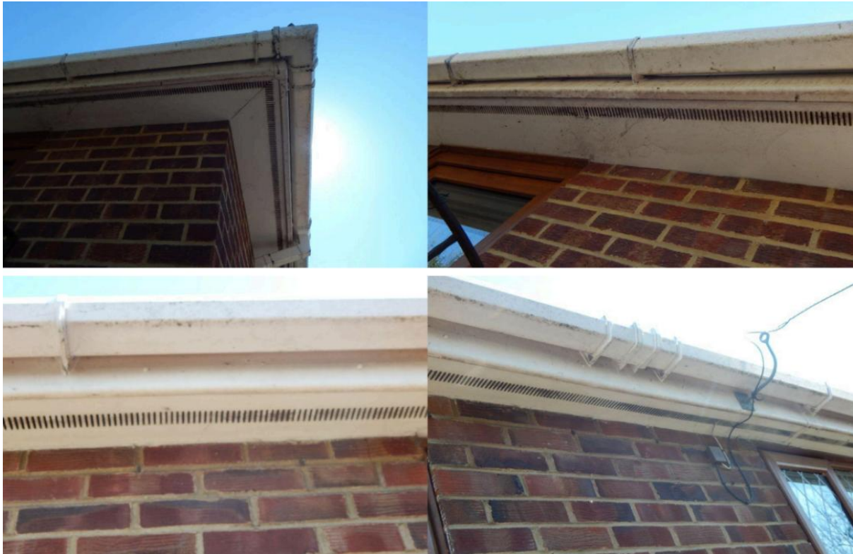
Image 7 – Close view of eaves coverings to demonstrate example of condition throughout
