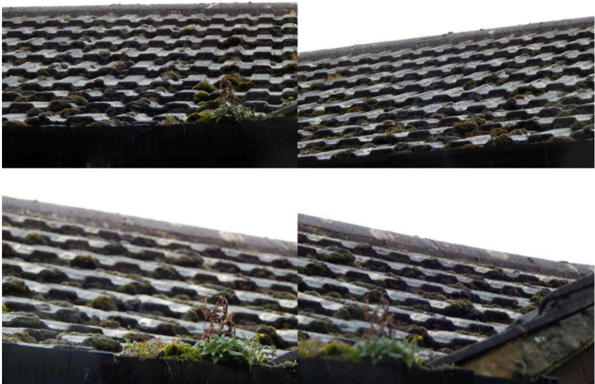
Image 4 – Views of the above roof coverings to demonstrate condition
