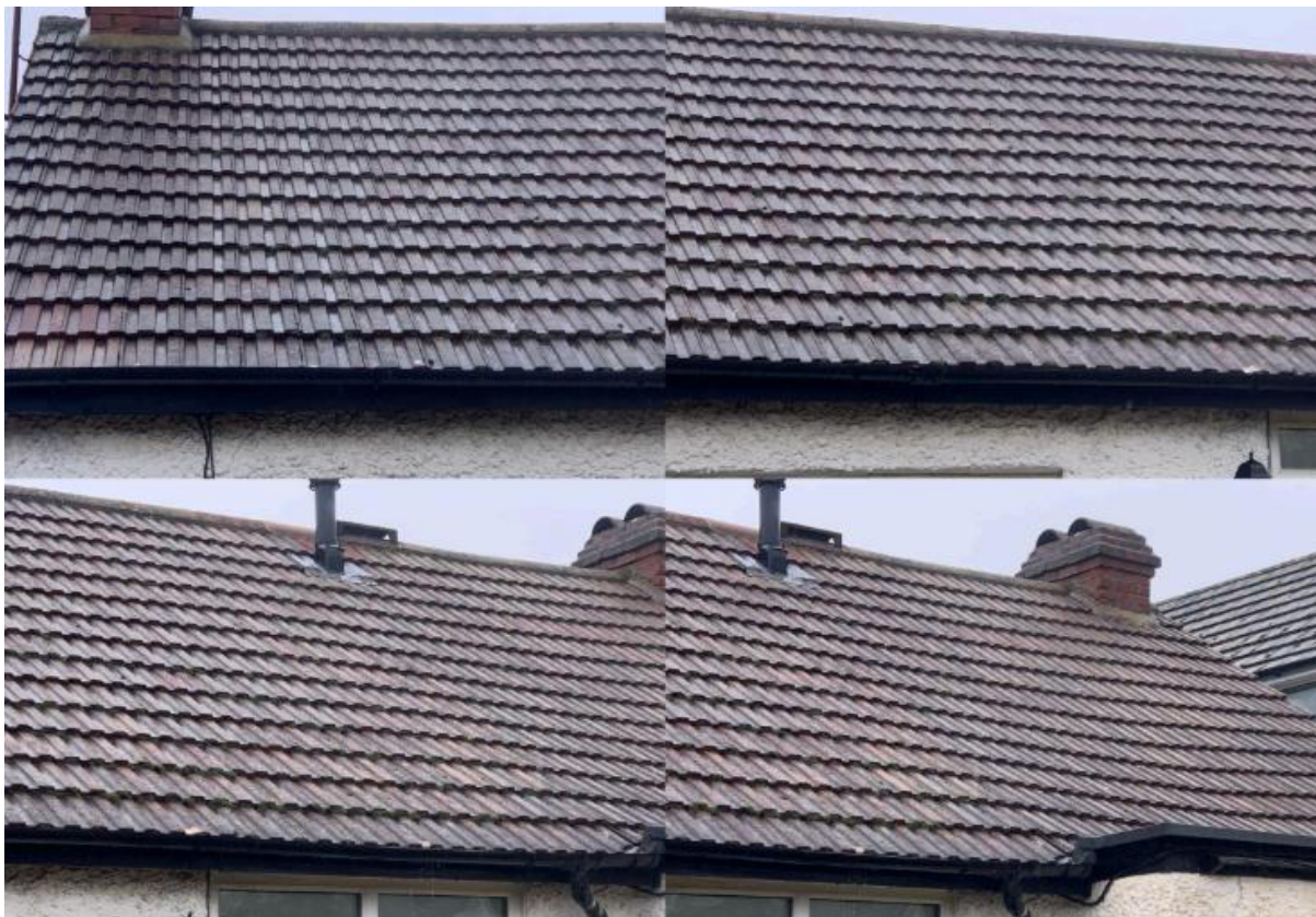
Image 2 – Views of the above roof coverings to demonstrate condition
