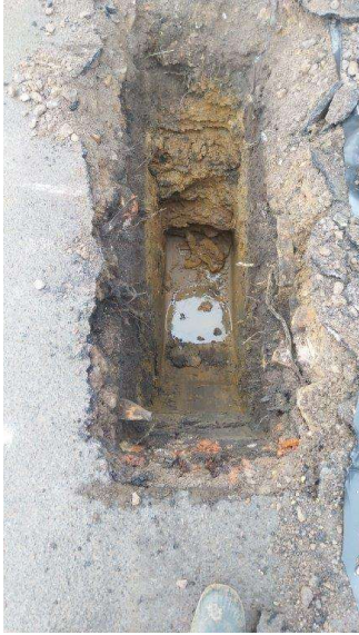
Photograph 7 - Looking down at water seepage encountered at 1.4m bgl within TP01.
