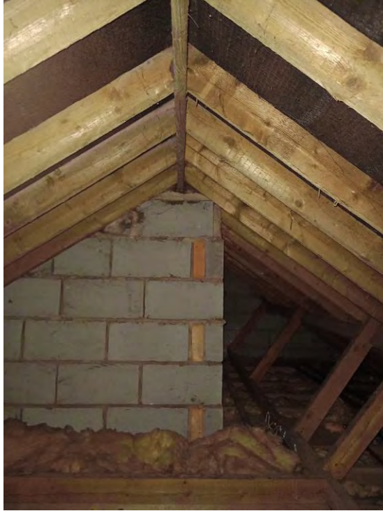
Figure 4: Void over the extension
