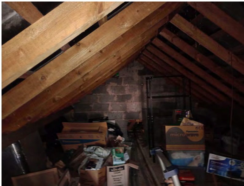
Figure 3: Void over the original building with hole leading to second void.
