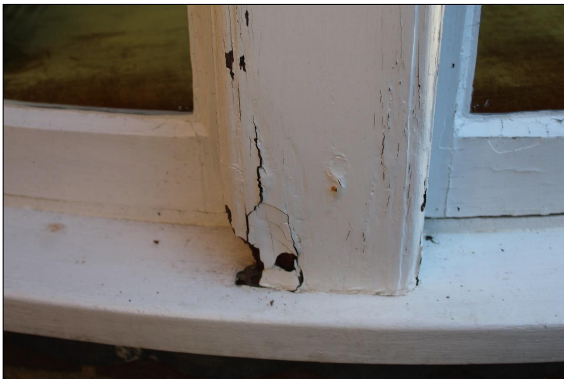
Photograph 7 – Areas of decay to the existing bay window
