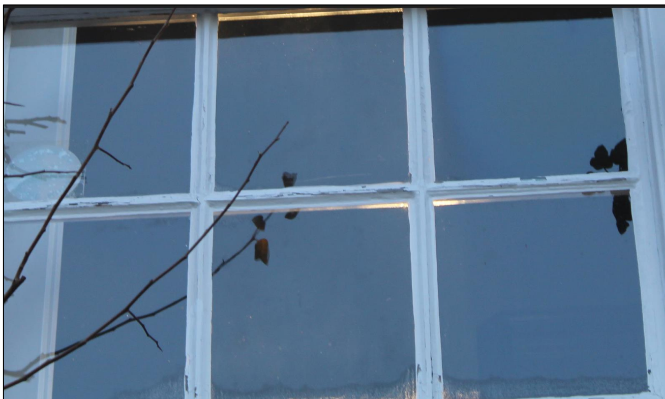
Photograph 6 –An example of the glazing bars to the existing windows. The damage to these profiles clearly visible in the above photograph.
