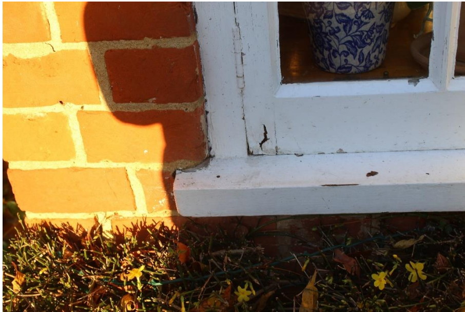
Photograph 8 – Areas of decay to the ground-floor rear elevation window
