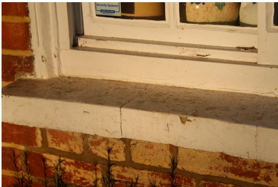
Photograph 9 – Areas of decay and cracked paintwork to the utility room Yorkshire Sash
