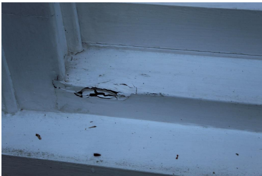
Photograph 10 – Areas of decay and cracked paintwork to the side elevation sash window
