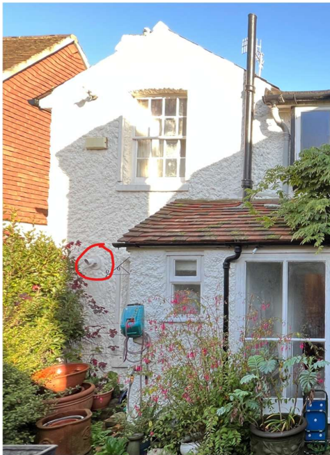
(Existing extraction vent highlighted in red)
