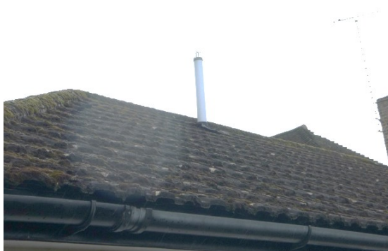
12. Gap beneath flashing around flue (western elevation).
