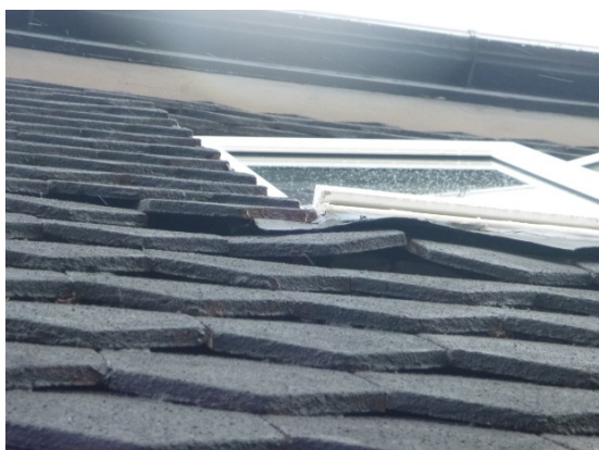
9. Slight gaps behind hanging tiles (front elevation).
