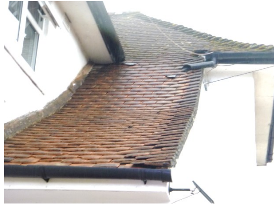
4. Occasionally lifted clay roof tiles along the verge (west elevation).
