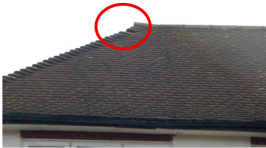
3. Missing mortar beneath hip tile (front elevation).
