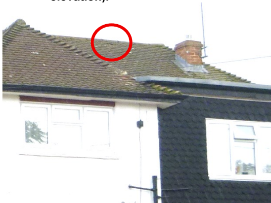
5. Missing roof tile beneath ridge (front elevation).
