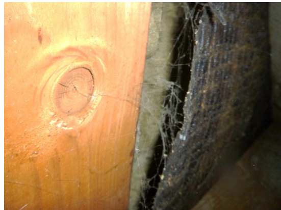
16. Dropping sections of bitumen felt with roof tiles visible.
