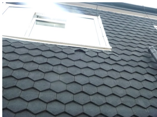
8. Missing hanging tile (front elevation).
