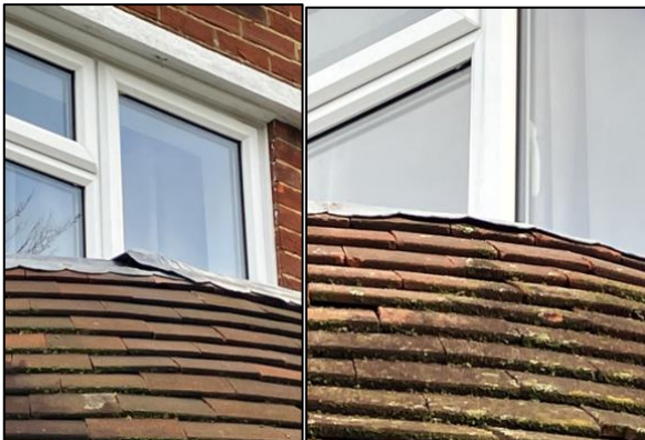
Photograph 3. Raised lead flashing on the roof of the orangery.
