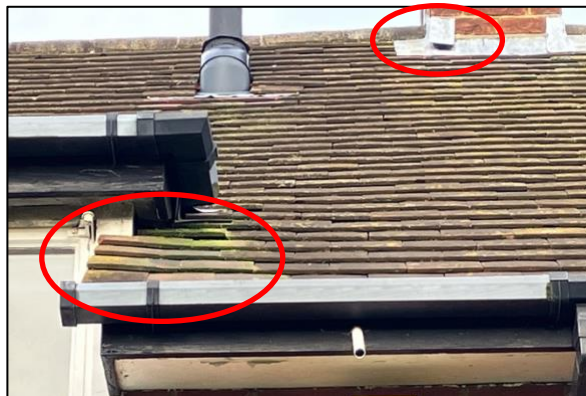
Photograph 4. Raised lead flashing around the chimney and slipped roof tile on the rear aspect.
