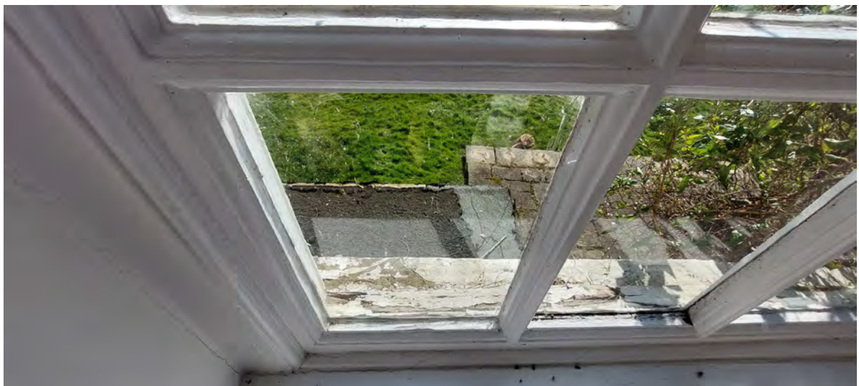
Example of poor condition of window cills
