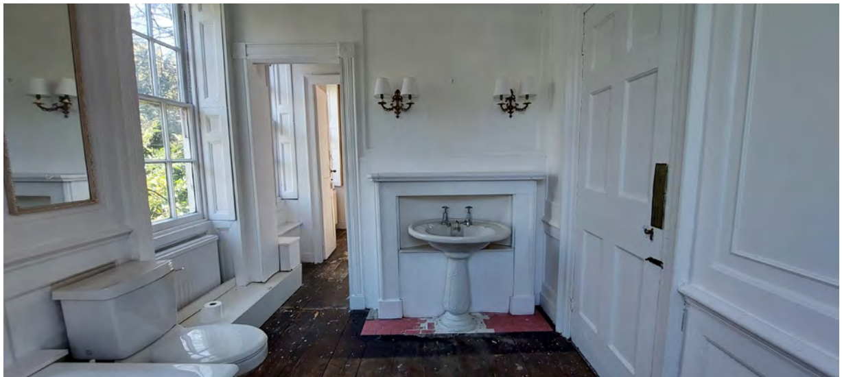
A number of alterations to the primary bedroom ensuite has resulted in a loss of historic features
