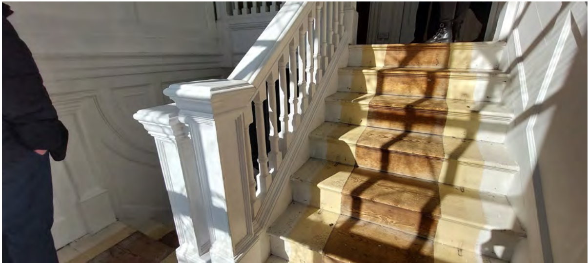
Evidence of changes to historic floorboards in main staircase
