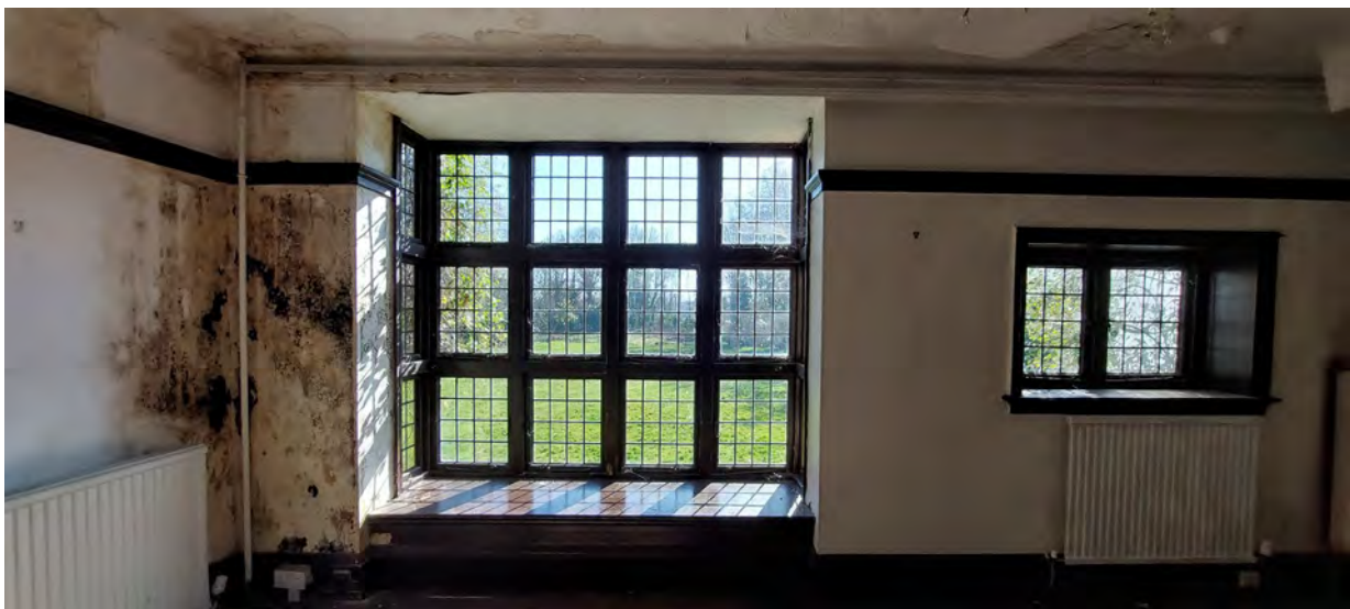
Severe mould and water ingress into ground floor drawing room; historic joinery and window
