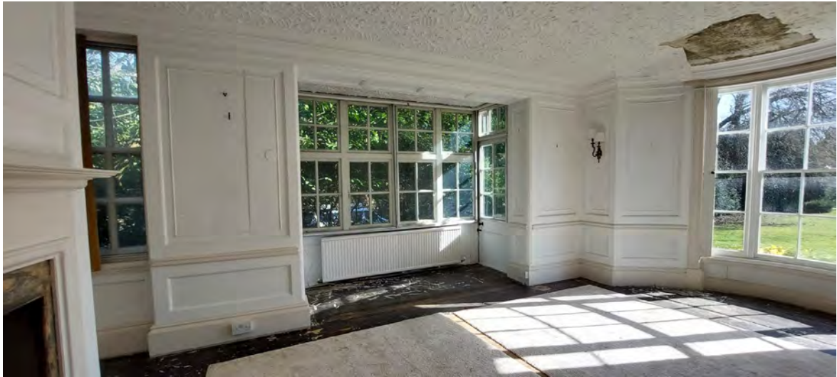
Damaged ceiling plaster in ground floor garden room
