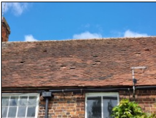
Figure 33 – Southern roof face of Rose Cottage with slipped roof tiles.
