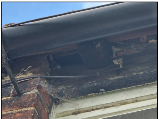
Figure 34 – Gap in the eaves above the northern elevation.
