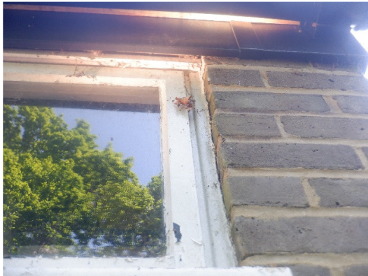
Photograph 9. Gap behind the barge board to the rear of the house.
