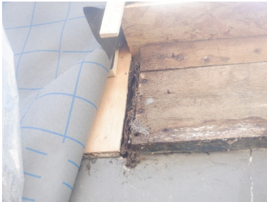
Photograph 3. Loose breathable membrane around the building.
