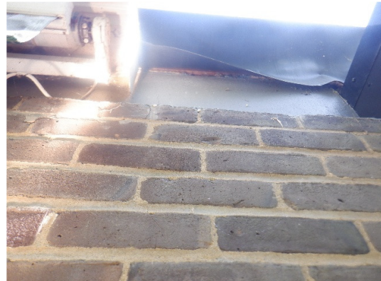
Photograph 10. Loose sheeting on the flat roof extension to the rear of the house.
