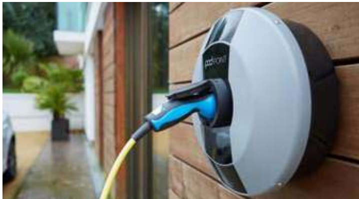
EV charging points fitted to all dwellings
