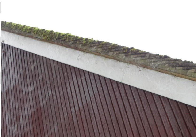
Photo 8: Tiles and fascia board at rear of property
