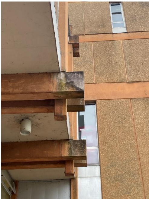
Photograph 19 – Vegetation growth on top surface of beam end tips (south elevation)
