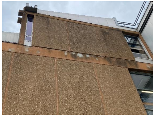
Photograph 16 – Previous concrete repair mortar repairs to concrete PT beam (level 3) on south elevation.
