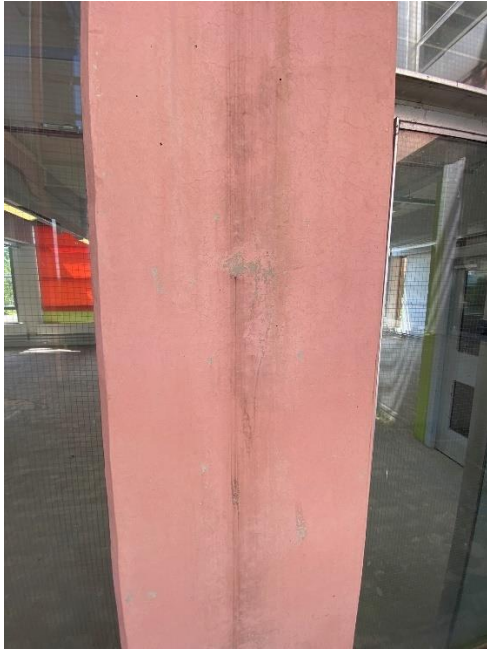
Photograph 33. Grazing cracks and peeling paint on level 2 columns within light well
