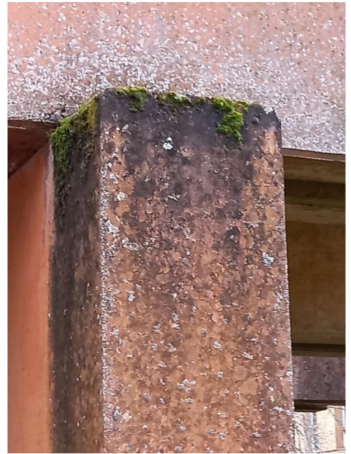
Photograph 18 – Moss and algae growth on concrete PT beam ends (level 1) on south elevation.
