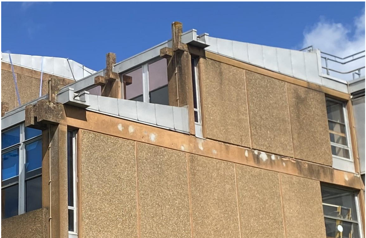
Figure 3 Poor quality previous concrete repairs on east elevation façade
