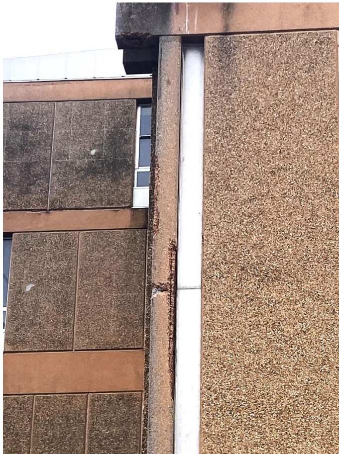
Figure 5 Spalling of exposed post-tensioned beam end
