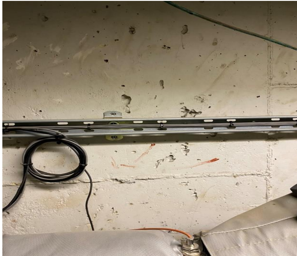
Figure 7 Honeycombing on internal face of basement RC retaining wall
