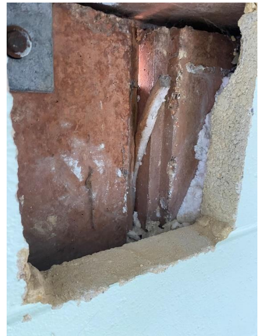
Photograph 20 – Failed mastic seals on precast cladding panels with daylight visible.
