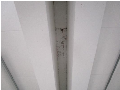
Photograph 43 - Poor compaction and honeycombing issues on slab soffit between PT double beams.
