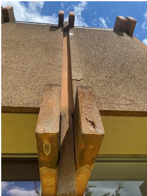
Photograph 7 - Concrete spalling on PT beam ends on south elevation level 1.
