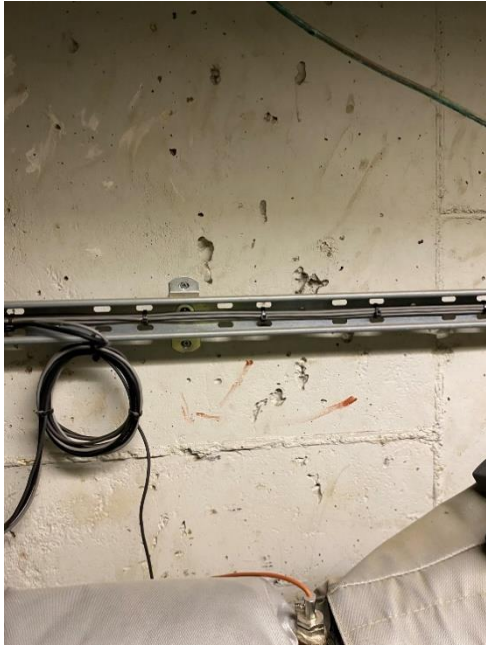
Photograph 41. Honeycombing on basement retaining wall
