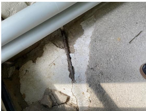
Photograph 25. – Damage to floor screed (50mm) on upper floor slabs
