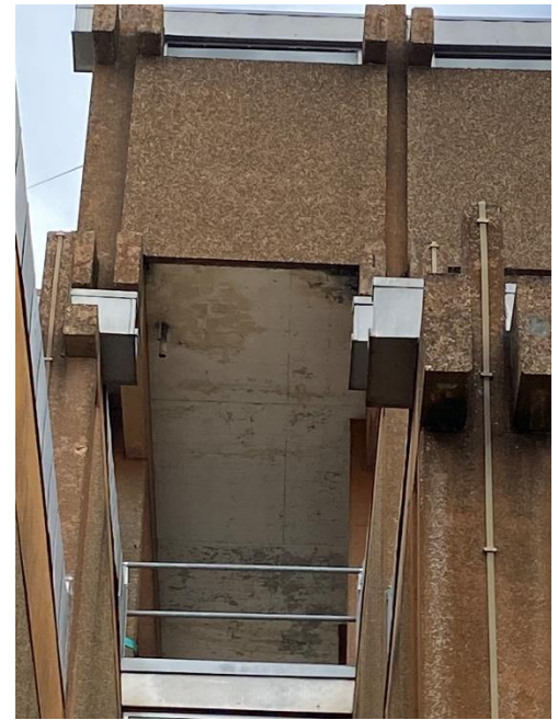
Photograph 12 – Water damage to insulation cladding panel boards located on overhang soffits.
