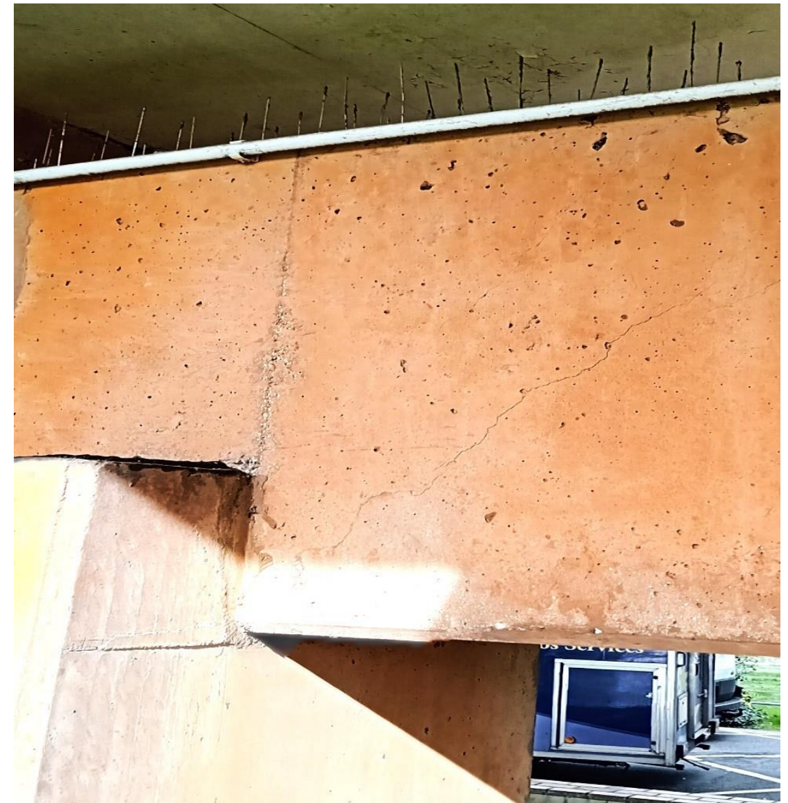
Figure 8 Diagonal cracking and honeycombing on RC transfer beam near external pond
