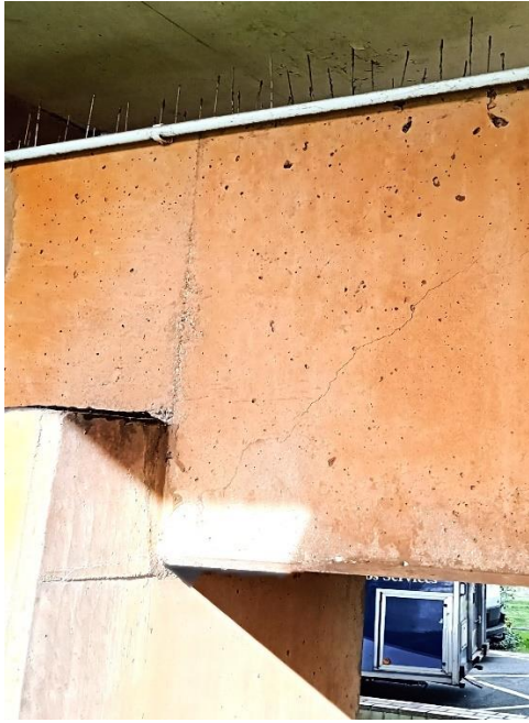
Photograph 17 – Diagonal hairline cracking on level 1 transfer beam above garden pond.
