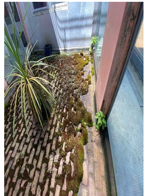
Photograph 32 – vegetation growth on level 2 roof surface within light well.
