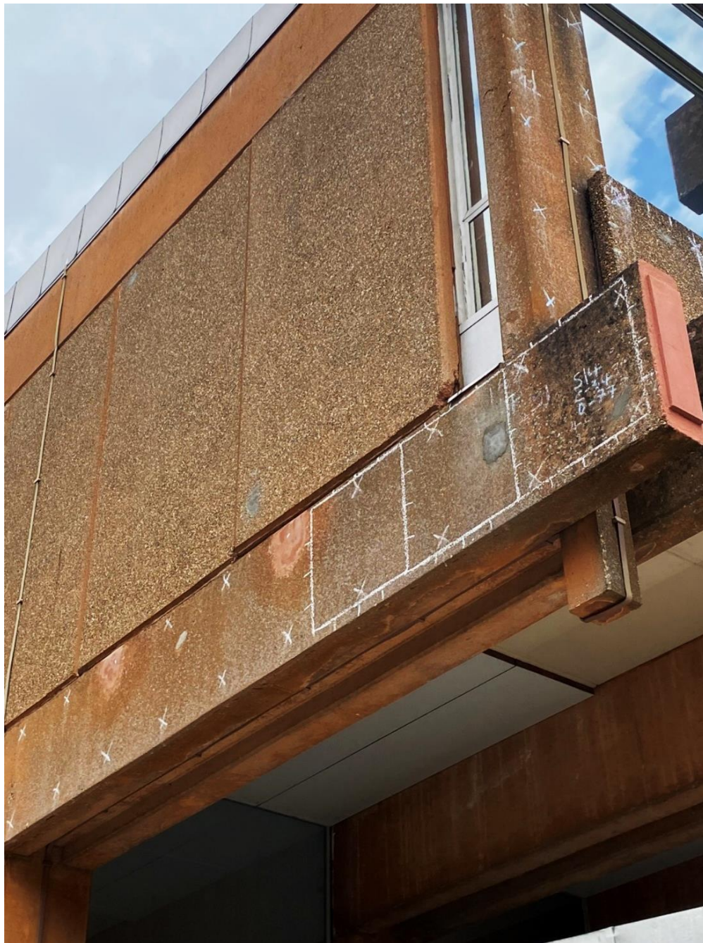
Figure 9 Out of plumb cladding panel above PT beam with hairline cracking at panel bottom edge.
