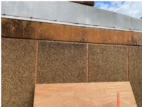
Photograph 15 – Moss and algae growth on beam and cladding panels (general comment).
