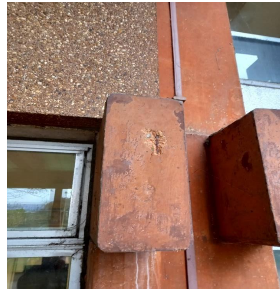
Figure 6 Steel reinforcement exposed on Post Tensioned RC beam end
