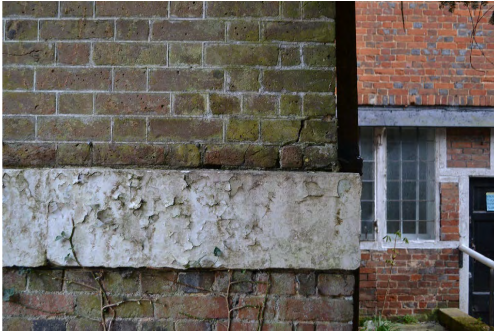
P25 Front right-hand corner – cracking
