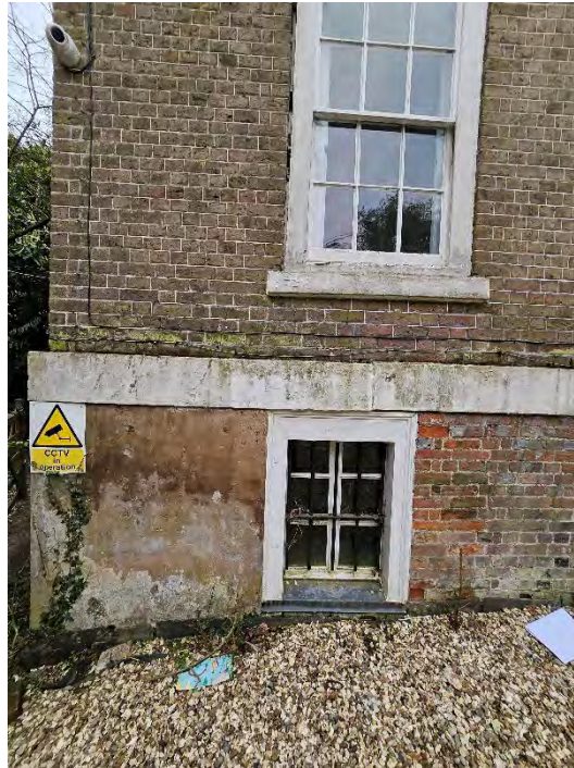
P35 Left-hand corner - movement above basement window
