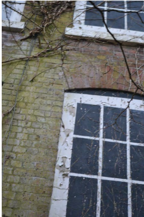
P37 Note displacement to arch
