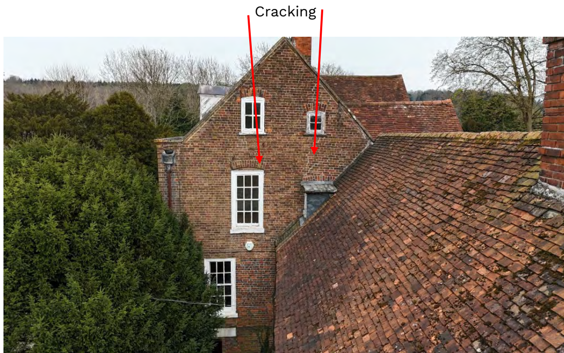
P31 Cracking to gable wall although previously repaired, continues to roof
