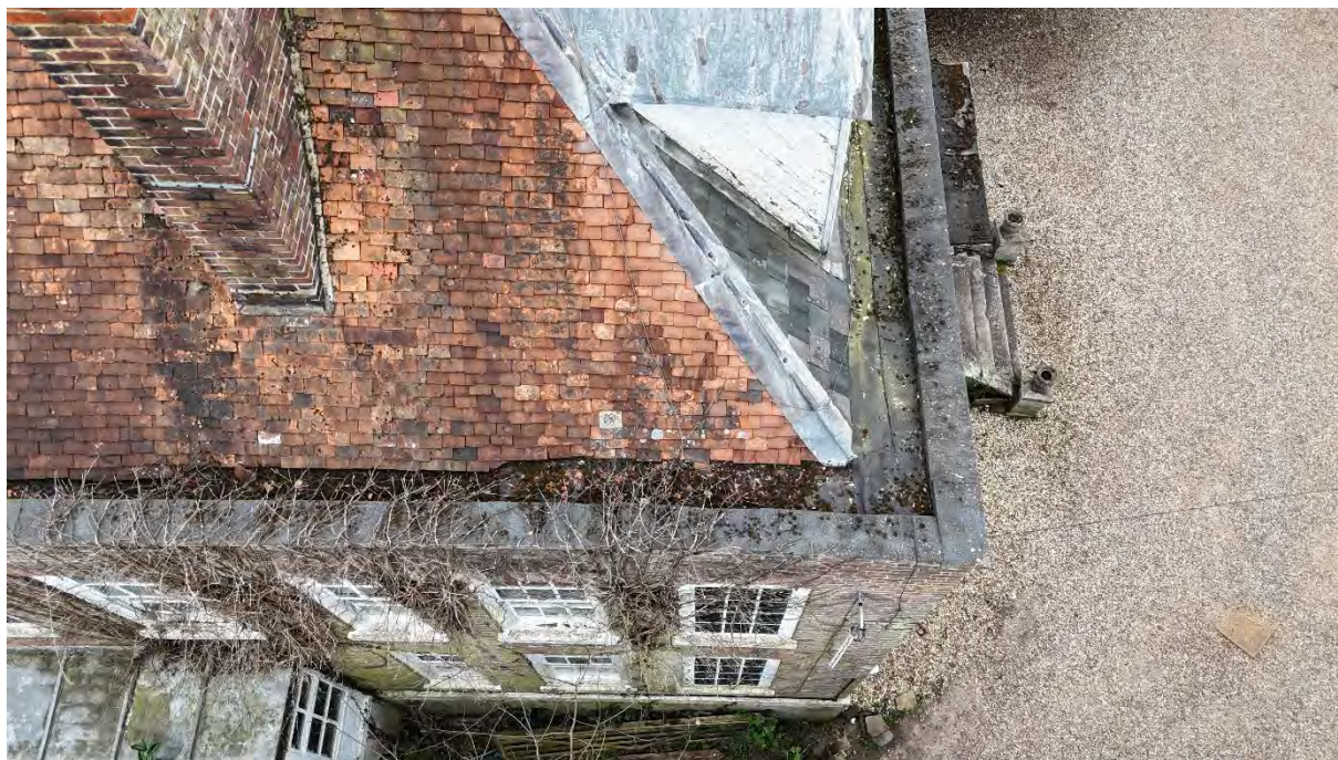
P21 Parapet gutters front and side
