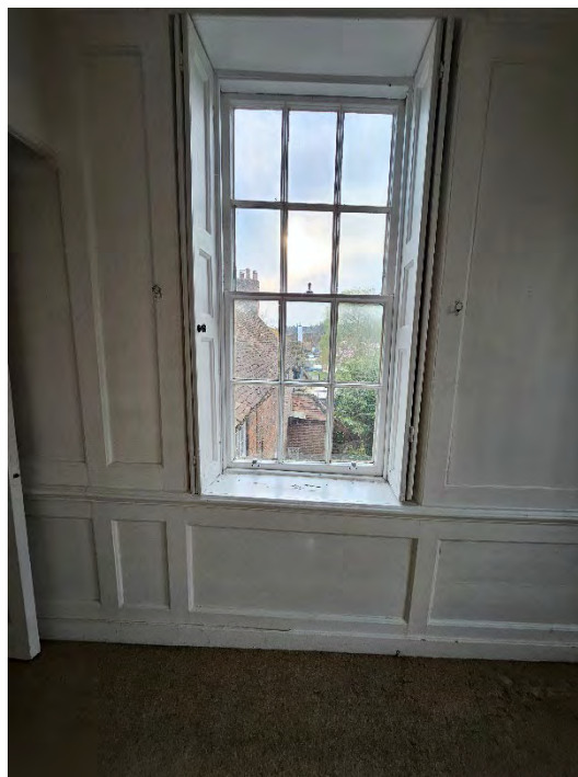
P74 First floor – right-hand gable – settlement to wall
