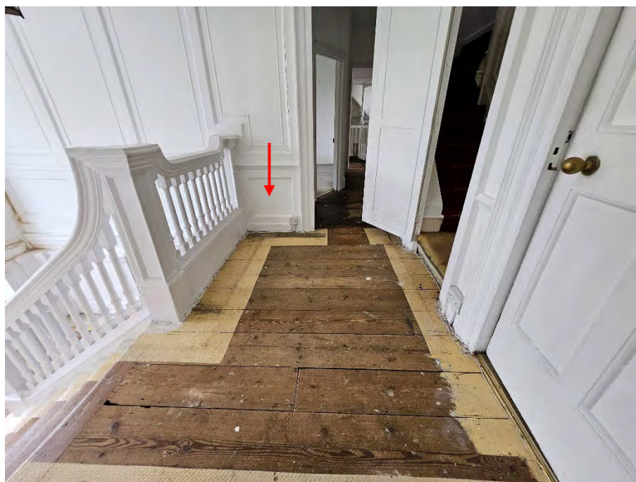
P72 First floor landing – slope to landing
