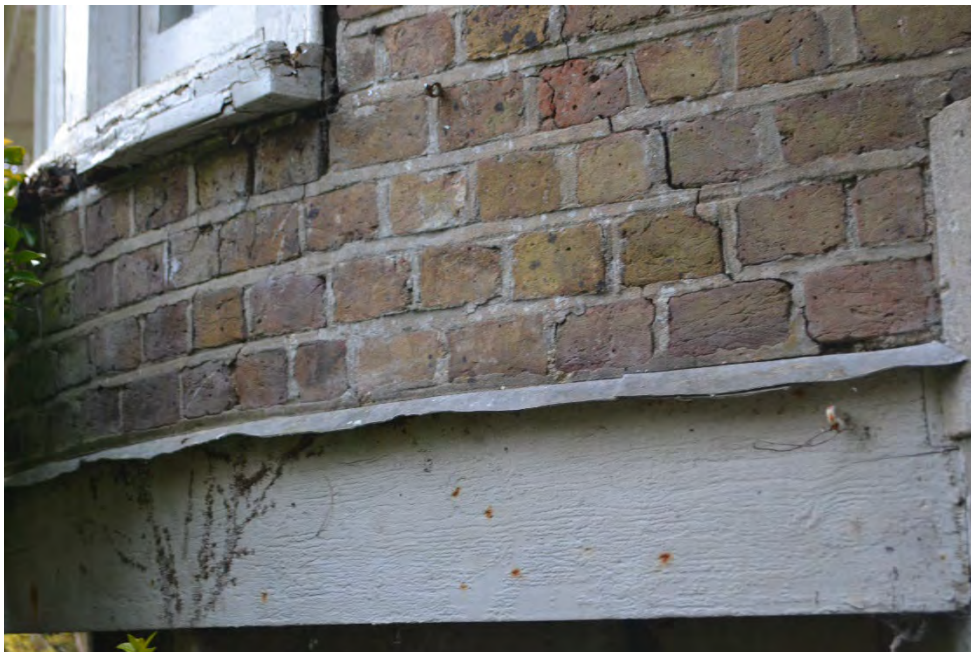
P40 Rear bay window ground floor – crack above ring beam
