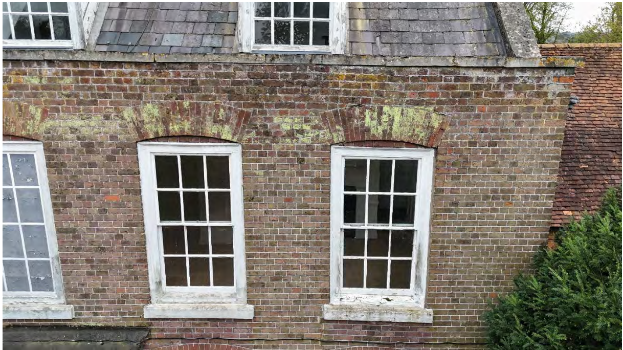
P27 Crack in front elevation continues to eaves
