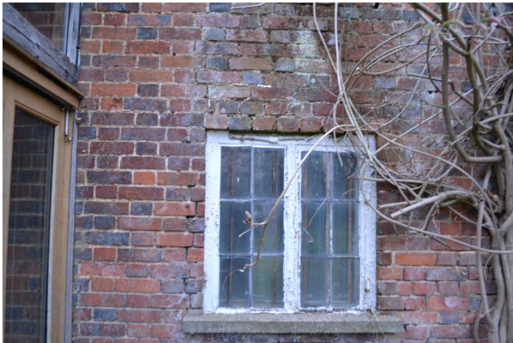
P48 Eroded and displaced brickwork
