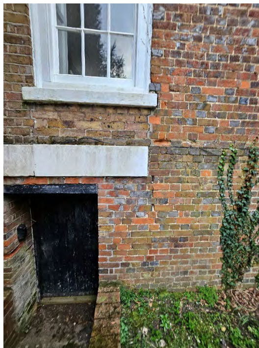
P28 Displacement to render course at basement door
