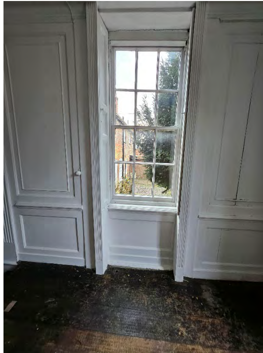
P63 Flank wall – front right-hand – cracking to panelling and distortion to window
