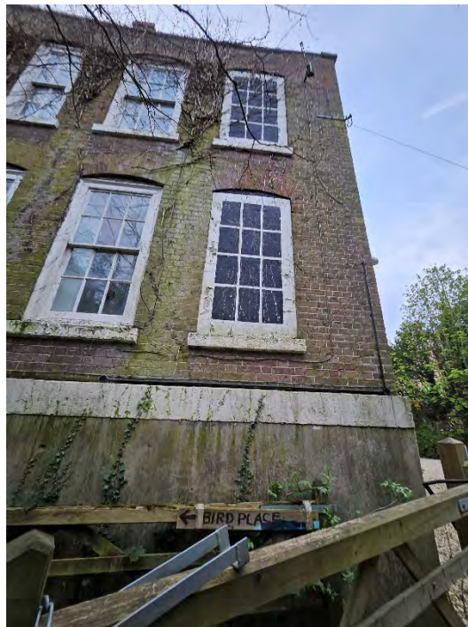
P36 Crack above window
