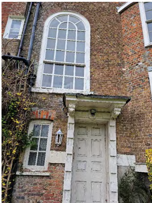
P43 Displaced brickwork above door
