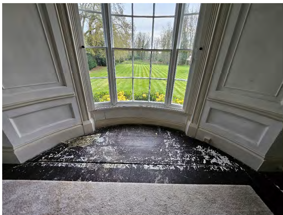
P68 Rear left-hand bay – note displacement at floor level
