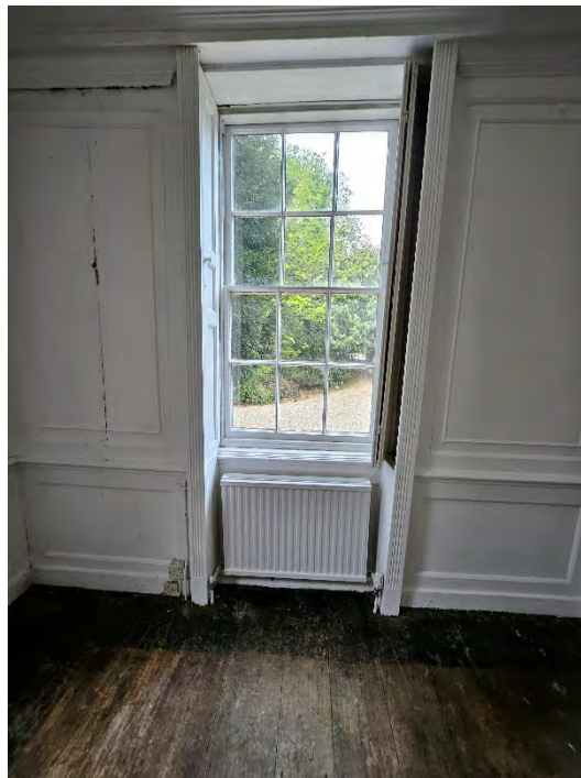
P62 Front right-hand corner – crack in panelling coincident with crack externally
