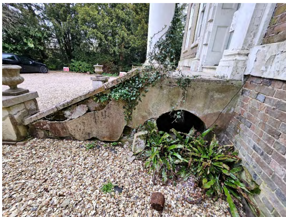
P31 Front steps – failed render
