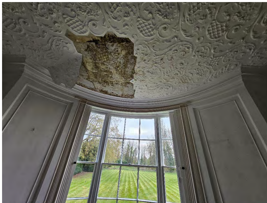
P69 Rear left-hand bay – loss of ceiling finish
