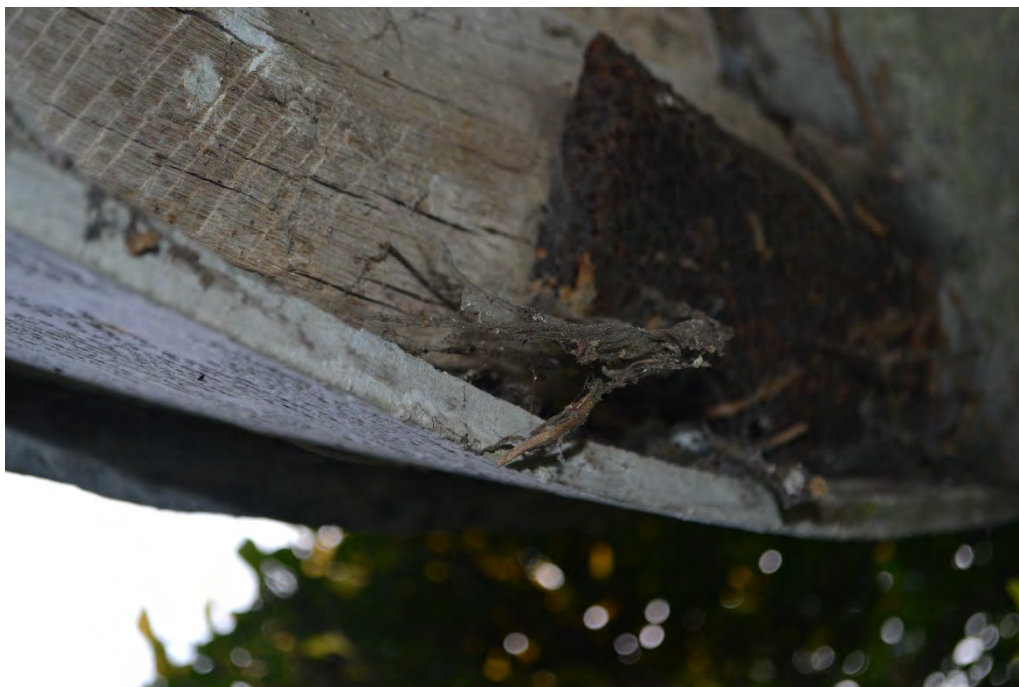
P41 Corroding steel in bay window support
