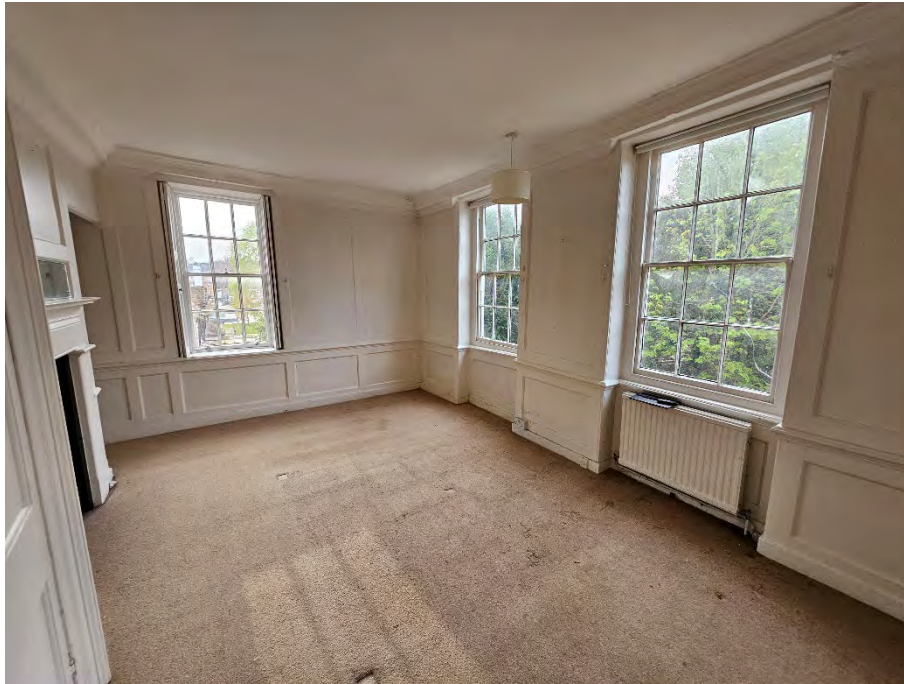
P73 First floor – right-hand corner – front. Note settlement to corner area.
