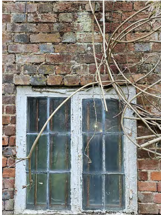
P45 Rose Cottage – rear. Displaced brickwork above window.
