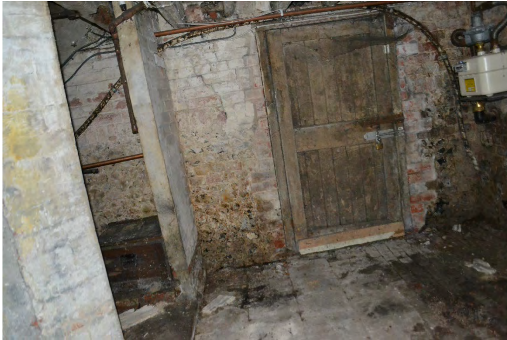
P49 External door – front right-hand flank wall into basement – note cracking
