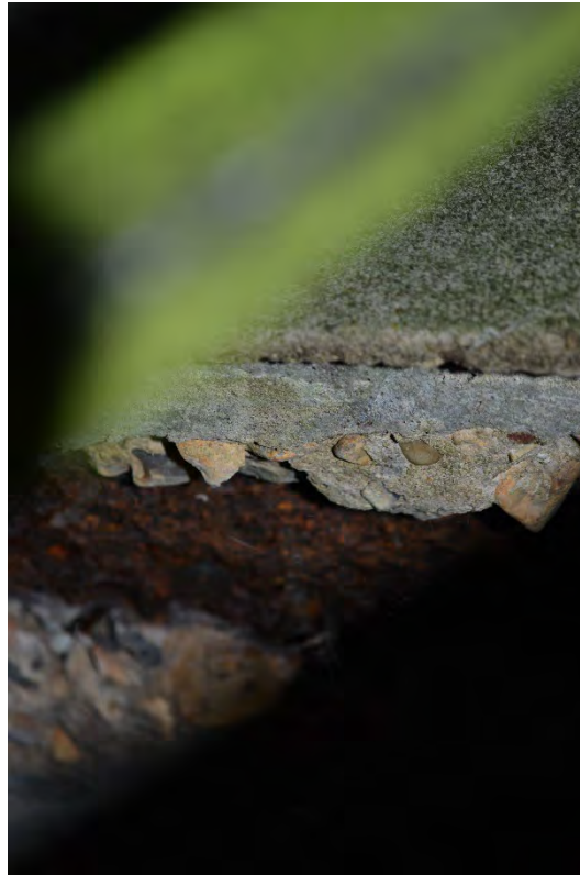
P39 Corroding steel below steps
