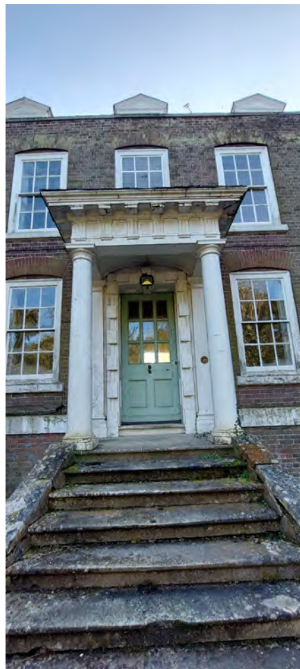
Main entrance, with deteriorated stone steps and modern half-glazed door
