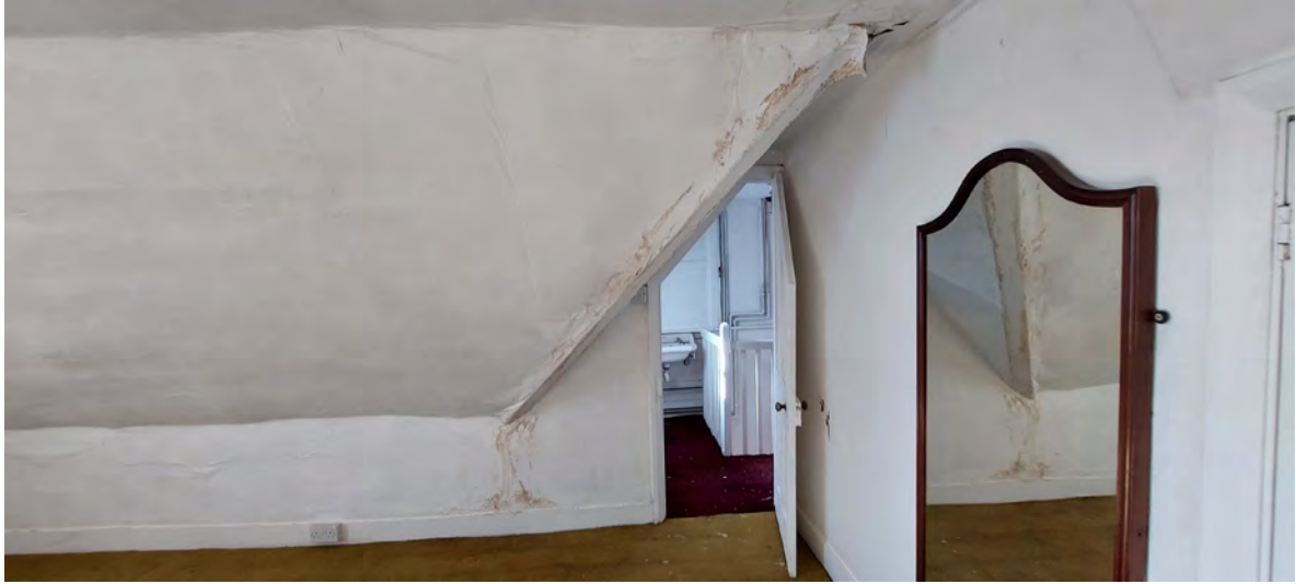
Water damage in attic room
