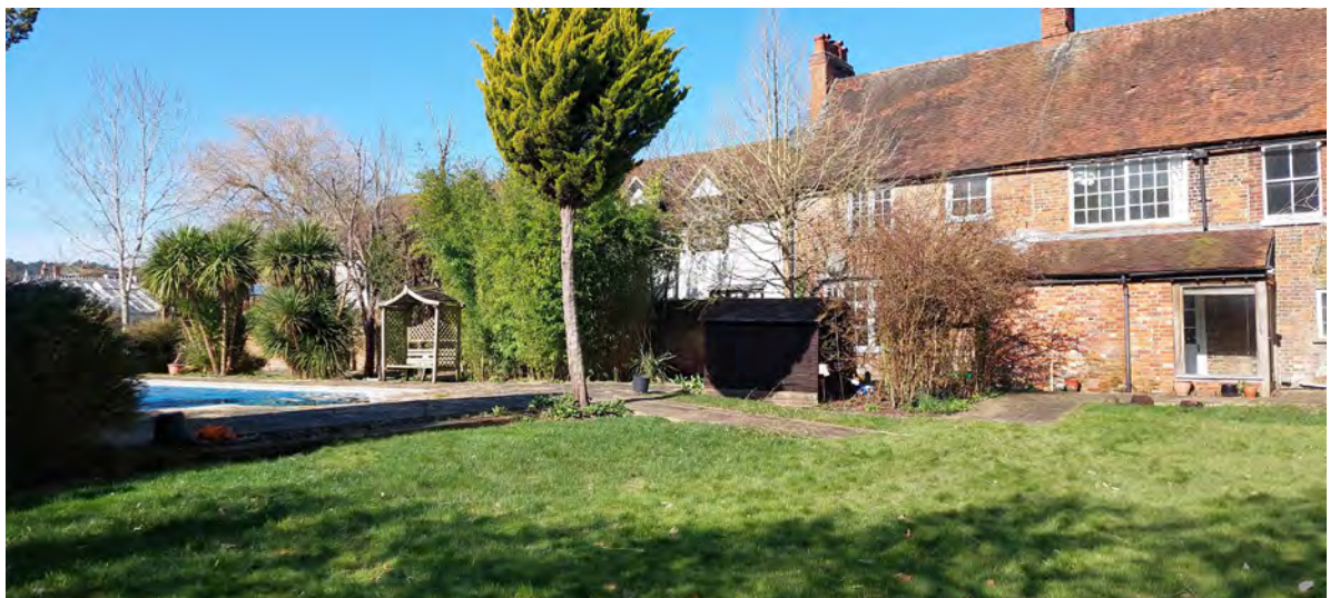
Poor-quality lean-to extending from Rose Cottage with Bird Place Cottage (white) to left behind brick wall
