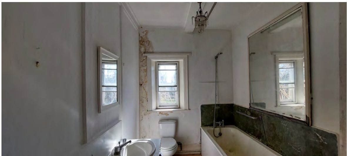
Historic flooring removed in bathroom; severe water damage
