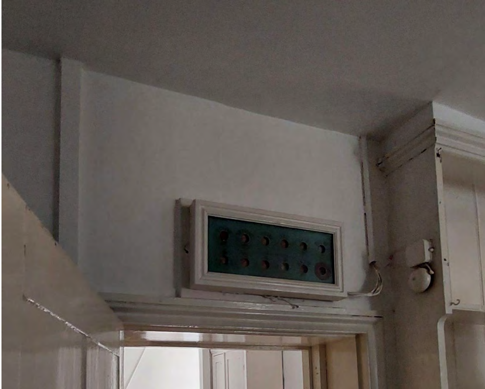
Historic service bell system in kitchen
