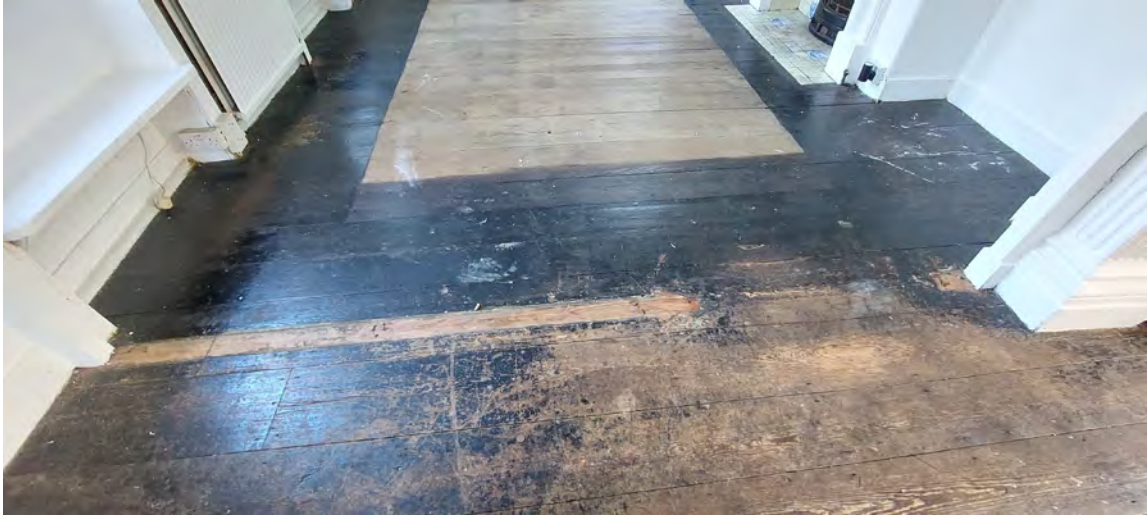
Evidence of possible former wall to room at left-hand side of ground floor entrance hall, with alterations to floorboards and dog leg walls
