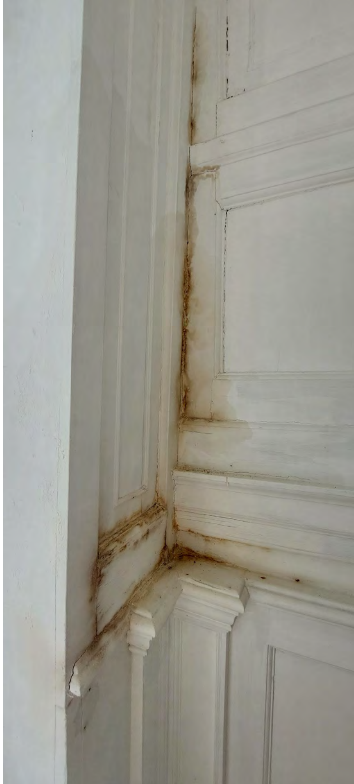
Water ingress in main staircase
