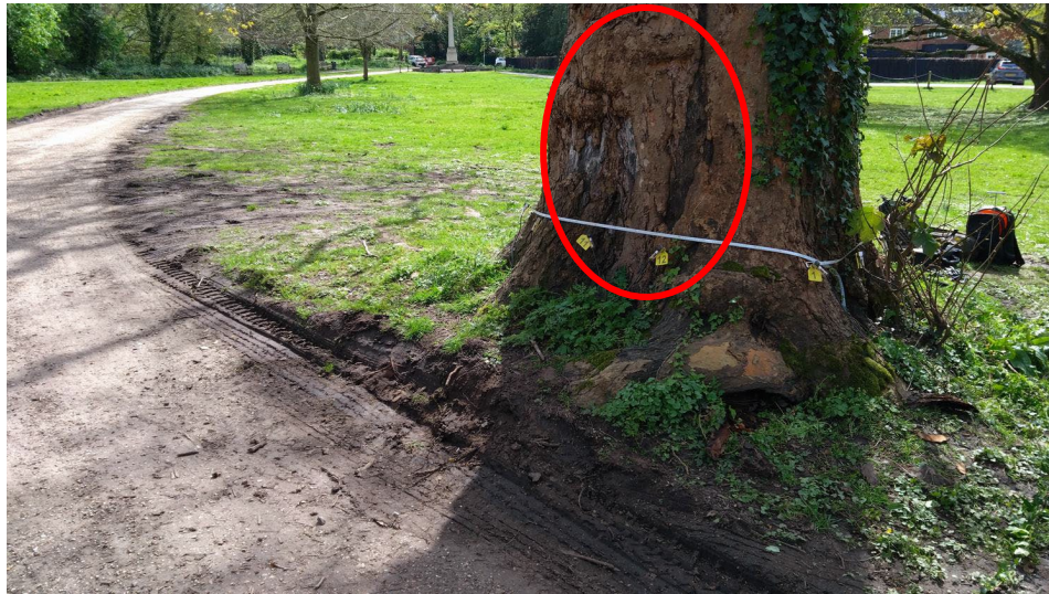
Figure 3: Void under eastern buttress (50cm probe fully inserted)
