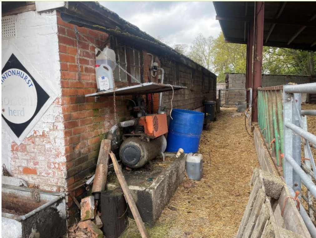
Plate 3 – View of small oil powered generator.
