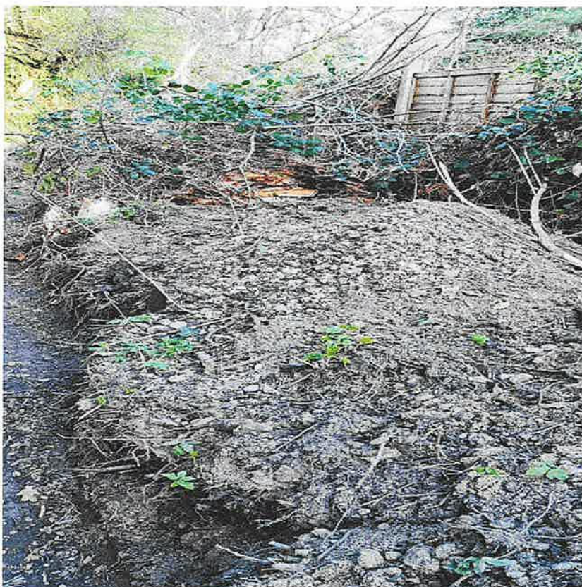
Picture 1 – Damage to Range Road near NMR
