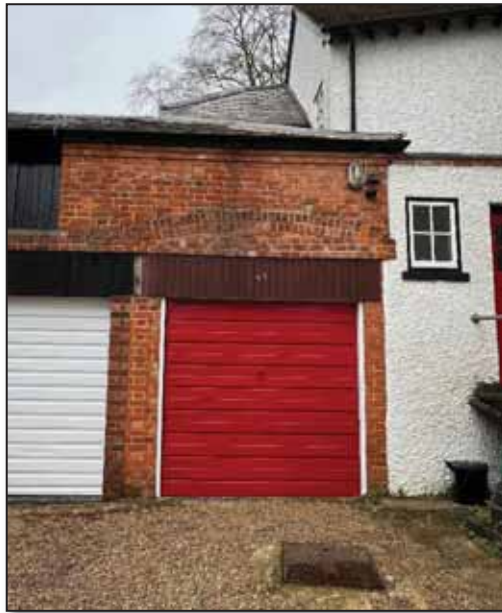
Image 14: Existing metal garage door
