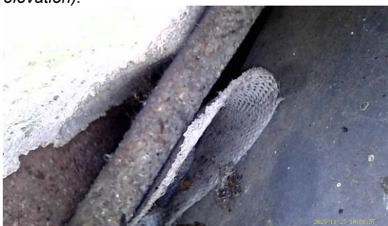
Photograph 5. Gap under tiles behind the chimney.
