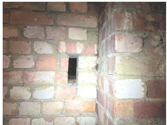
Photograph 17. Gap within party wall.
