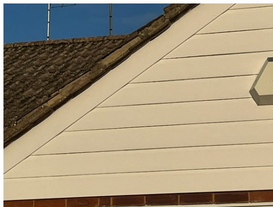
Photograph 8. Superficial crevice between mortar and under cloaking (front elevation).
