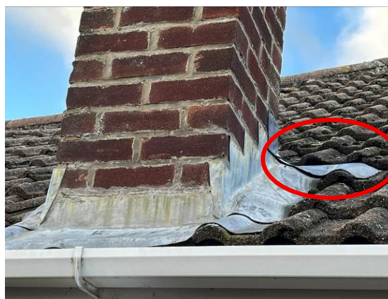
Photograph 4. Lifted interlocking roof tiles by chimney (southeast elevation).
