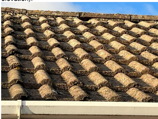
Photograph 9. Crumbling ridge mortar (southeastern elevation).
