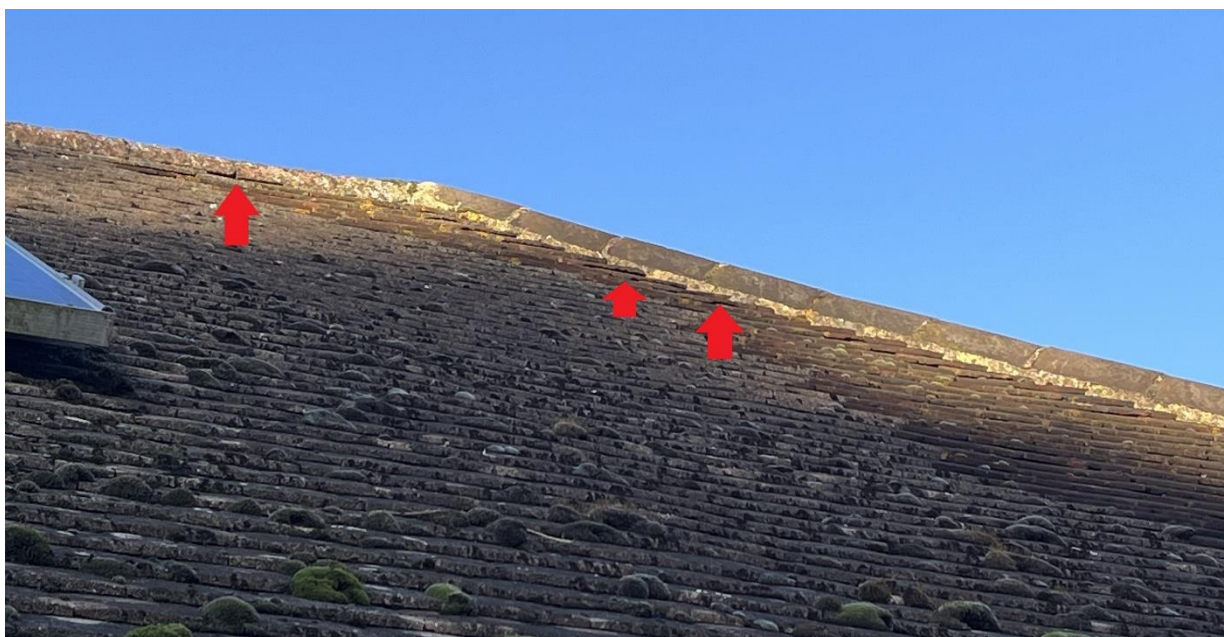
Figure 7. Detail of south face of roof looking east: red arrows indicate potential openings into undertile spaces
