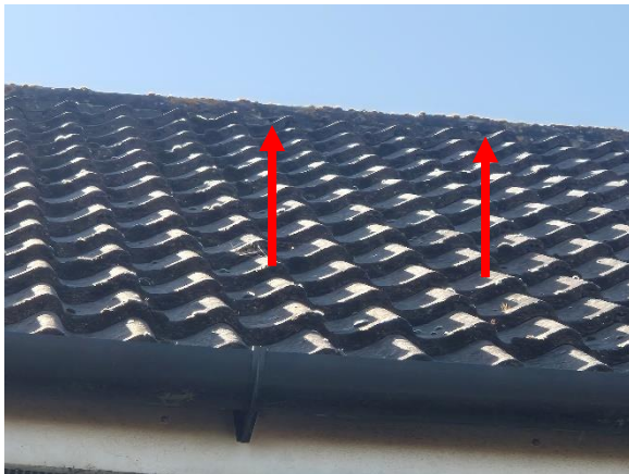
Photograph 12: Gaps at the ridge on the northern elevation of B1.
