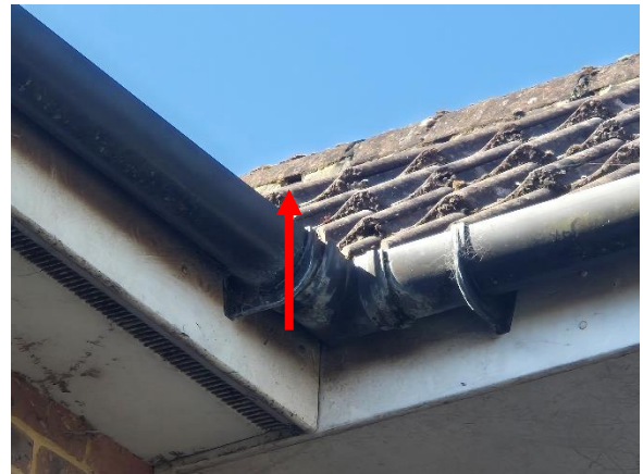
Photograph 13: Gap at the ridge of the dormer window on the northern elevation of B1.
