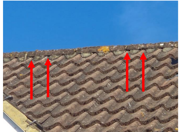
Photograph 11: Gaps at the ridge on the southern elevation of B1.
