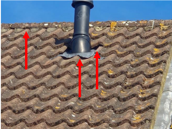
Photograph 10: Gaps at the ridge and around the vent pipe on the southern elevation of B1.
