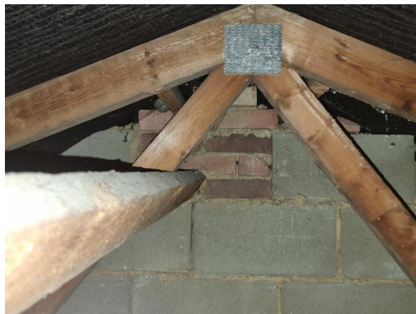
Figure 6. Gaps in interior gable wall.
