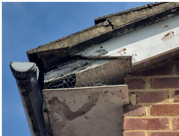
Figure 2. Gap in soffit box where it meets fascia. Gap has been covered by wide-spaced mesh.
