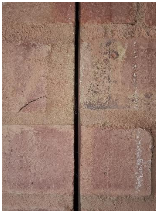
Figure 8. A sawn cut in the interior brick of the garage, which created an access point into the cavity wall. A similar cut existed within the brick in the main house, in the same general location as the cut in the garage. The cut in the main house also facilitated access into the cavity wall.
