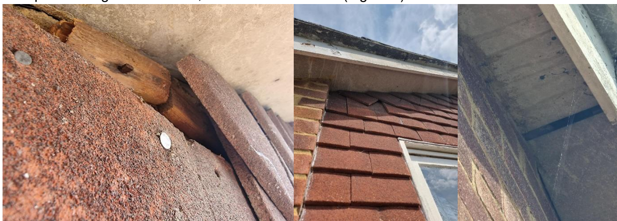
Figure 3. Gaps between hanging tiles, and gap in soffit at apex of gable end.
