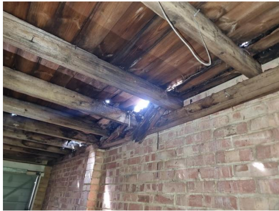
Figure 7. Garage interior with area of caved in roof.
