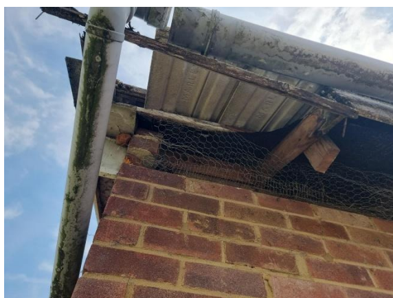
Figure 4. Damaged soffit covered with wire mesh.
