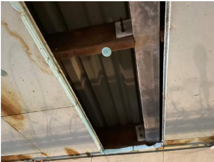
Missing polystyrene panel
