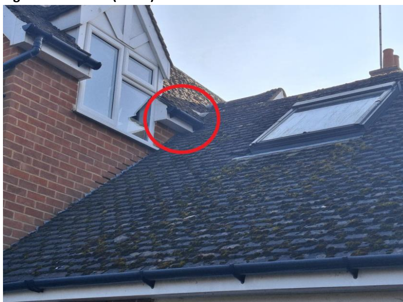
Figure 6: The rear (north) side of B1c. A red circle indicates the area of lifted lead flashing and soffit box
