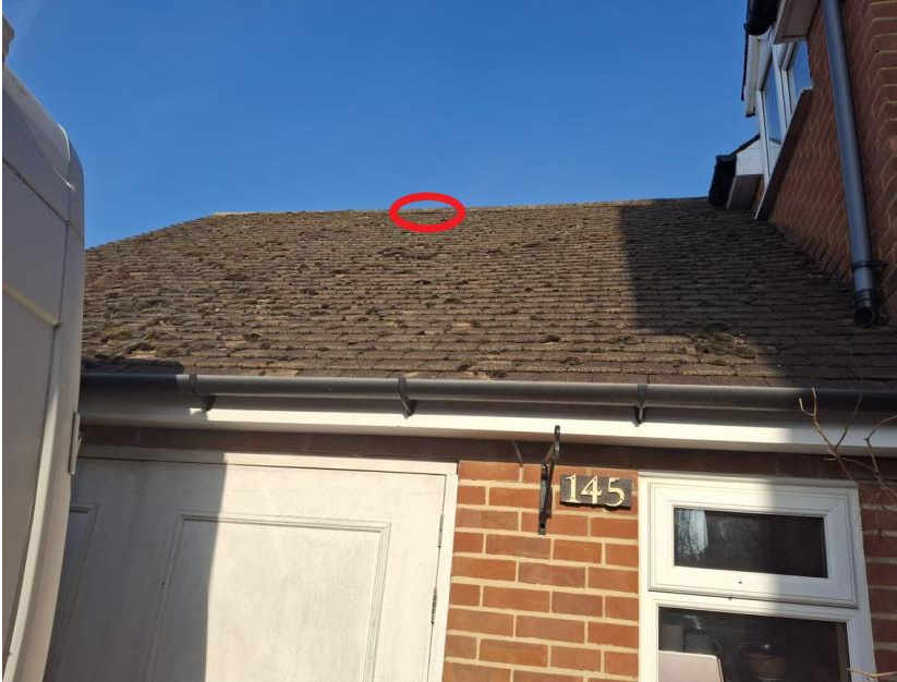
Figure 7: The front (south) side of B1c. A red circle indicates the lifted tiles below the ridge.
