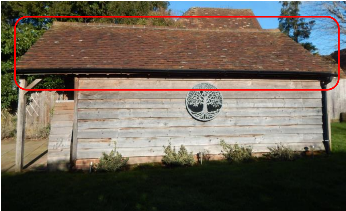
Image 3 – South facing elevation of the structure which has demonstrated a moderate number of gaps of adequate proportions across the tiled roof coverings offering likely shelter/access opportunities for bats
