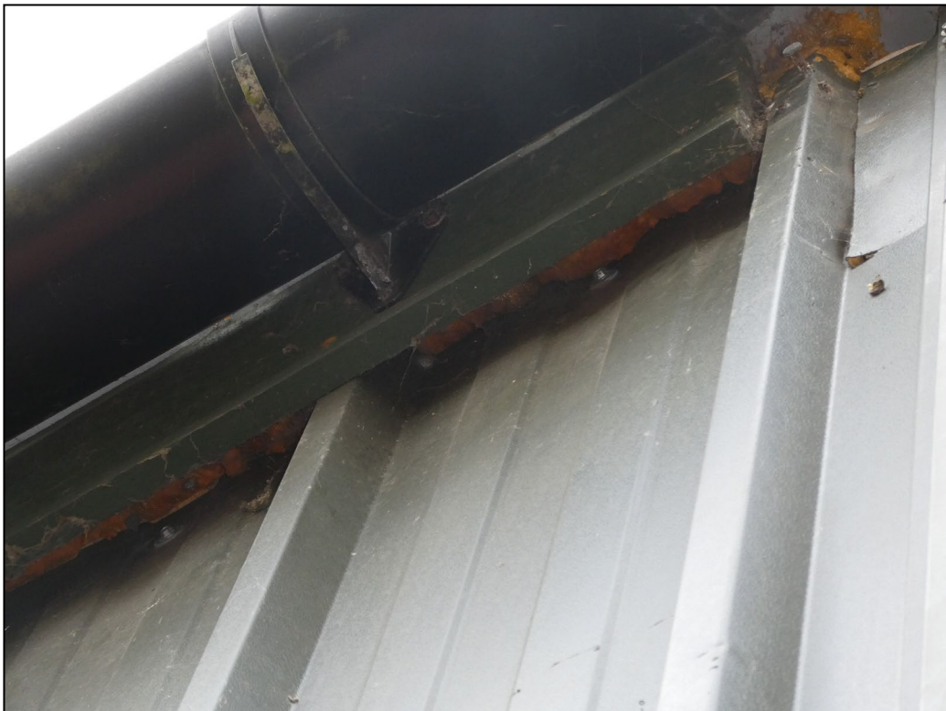
Figure 6. Example filled external gaps. Workshop at Springfields, Trowes Lane, Swallowfield. 01.02.23
