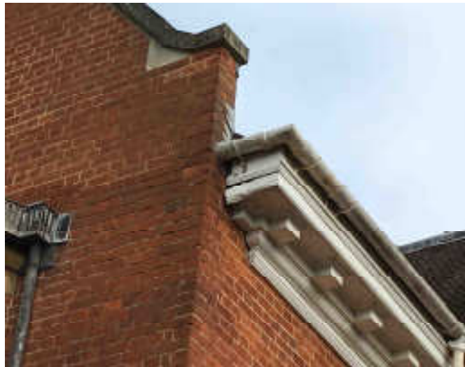
Indicative high-level defect
