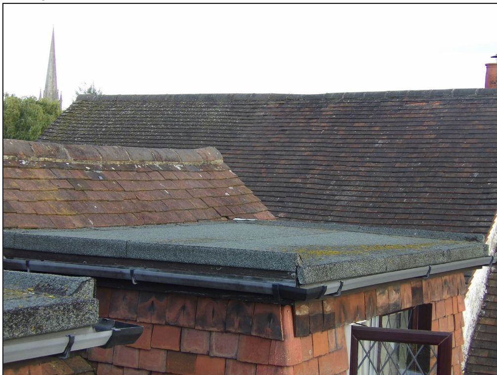
Figure 9. Example well fitted bitumen felt on dormer windows. 73 Oxford Road, Wokingham. 04.11.25
