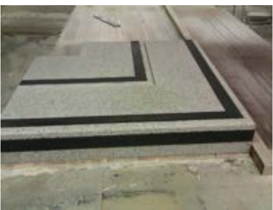
Marshalls Conservation X Step, coping stone to pond wall
