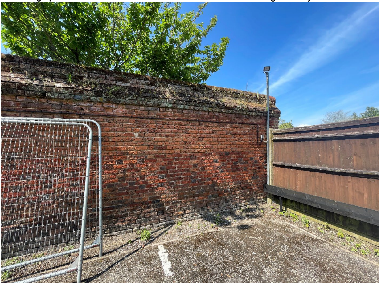
Photograph 4 - View of wall from southeast – corner to NE is propped by adjacent fence post
