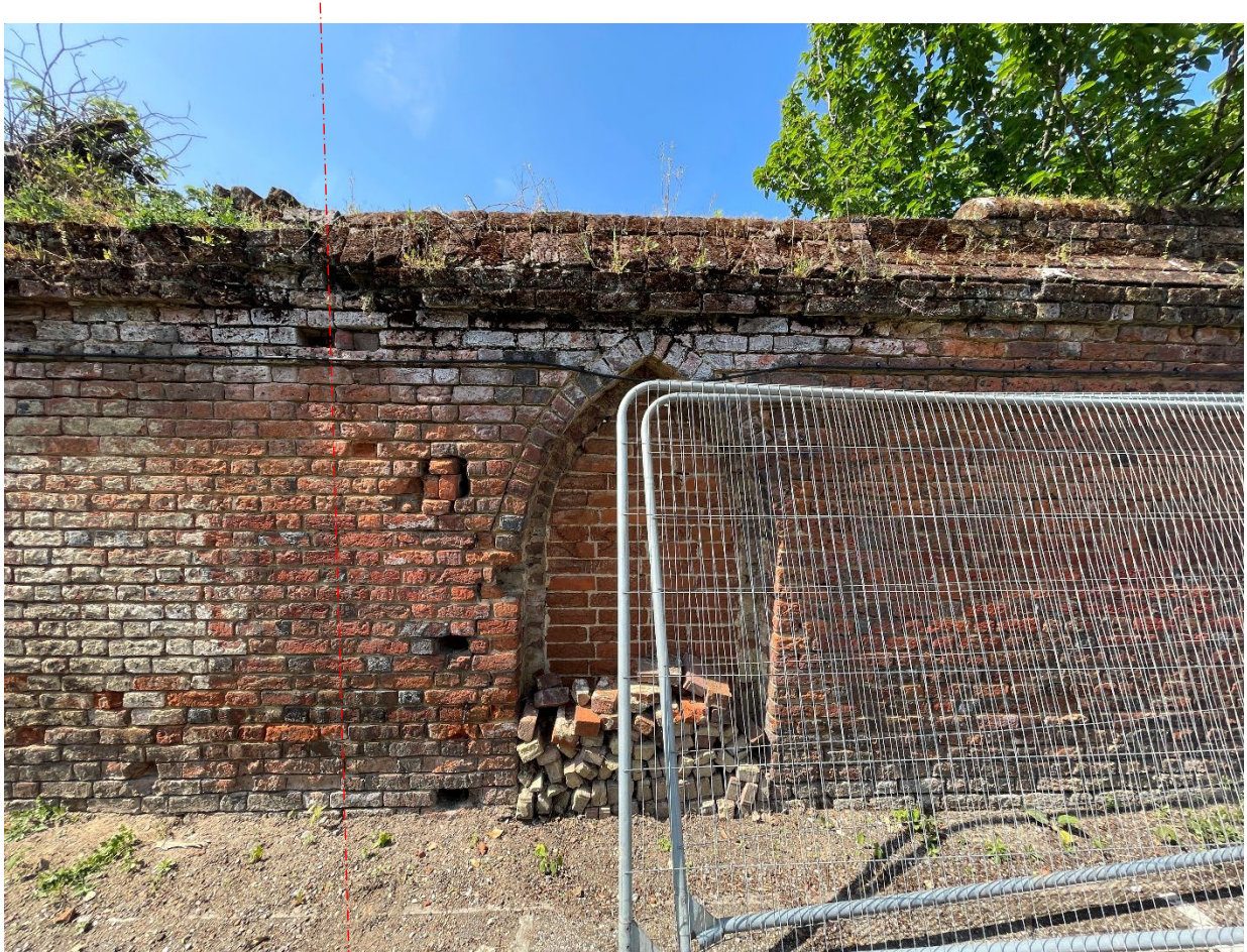
Photograph 3 – View of wall from southeast – wall starts to lean significantly to RHS of line
