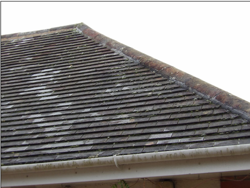
Figure 6. Example of ridge/hip tiles. 108 Reading Road, Woodley. 10.01.25
