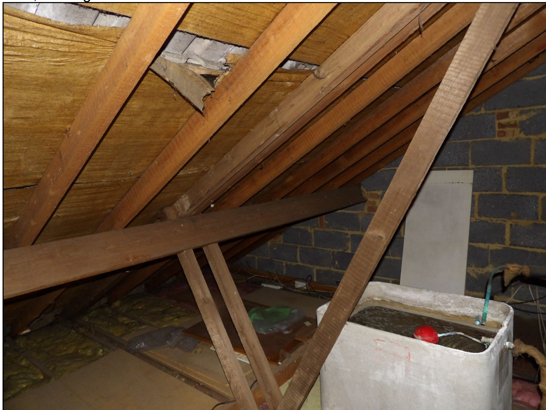
Figure 12. Example loft space and torn tar paper lining to tiles. 155 Old Woollah Lane, Wokingham. 22.07.25
