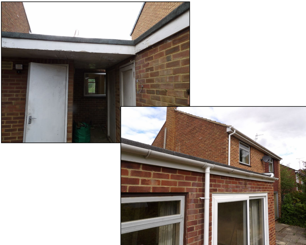
Figure 11. Example sealed fascias on link-attached garage/walkway/room. 155 Old Woosehill Lane, Wokingham. 22.07.25
