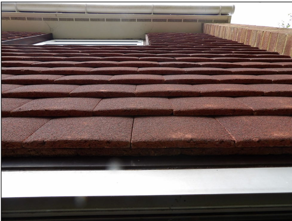
Figure 8. Example well fitted hanging tiles. 155 Old Woosehill Lane, Wokingham. 22.07.25
