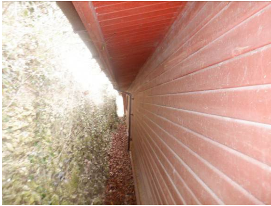
Photograph 5. Tightly fitted cladding on all sides (viewing eastern side)
