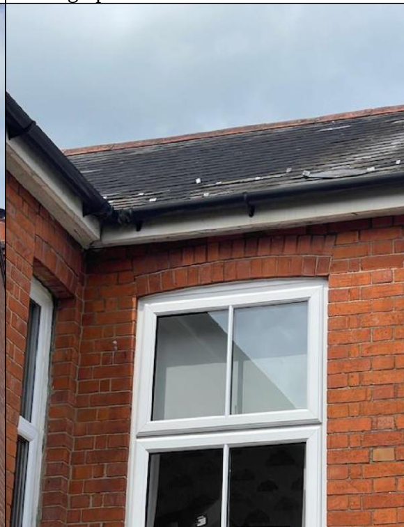
Photograph 4: Gaps around wooden soffits.
