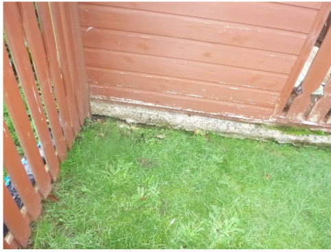
Photograph 11. Small gaps under a shed in the rear garden.
